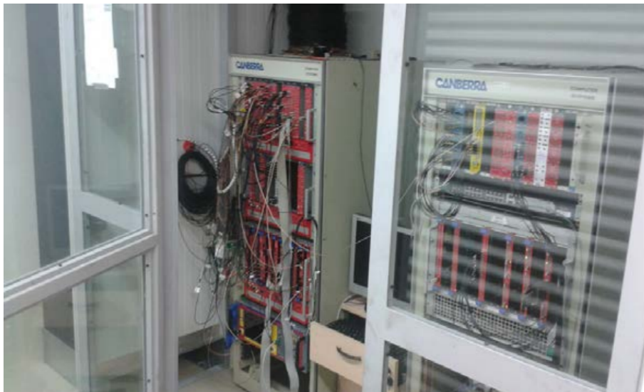
Figure 2.11: Temperature controlled room for ANAIS electronics at Hall B of LSC.
