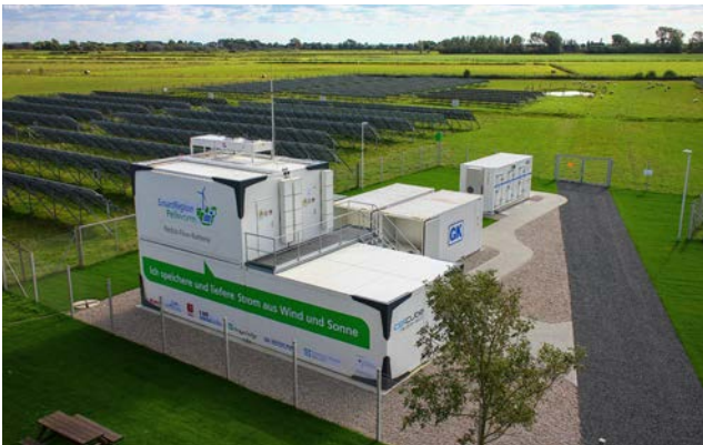
© E.ON. Hybrid storage system combines a redox flow and a lithium ion battery to provide high energy and high power.
