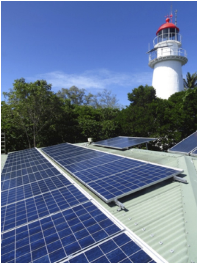
© Great Barrier Reef Marine Park Authority. Solar array 24 x 250W PV modules.
