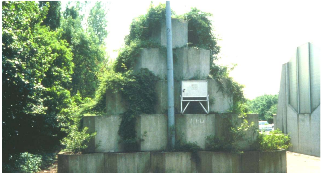
Figure 3.22. Supported earth embankment made of concrete pipes piled on top of each other in triangles and filled with earth along Highway A3 near Cologne in Germany [3].
