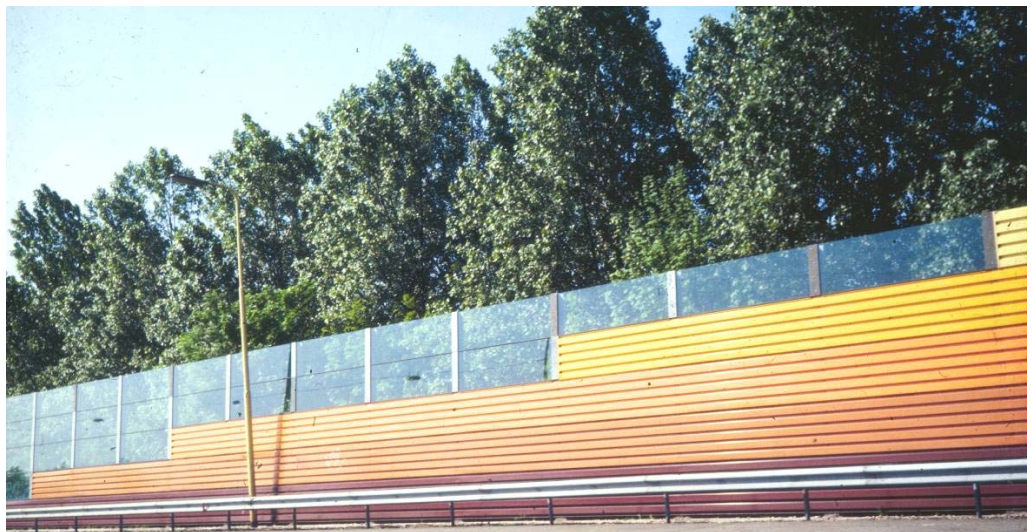
Figure 3.10. 4.5 m (15 ft) high noise barrier with light yellow color at the top and dark red colors below. There is a transparent part and high vegetation behind this barrier at Highway A9 in the Netherlands [3].
