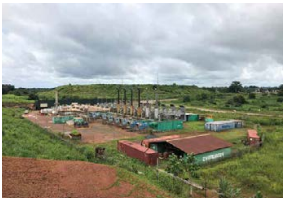
The Marampa project power plant, which will need complete overhaul before restart
