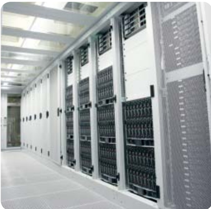
Figure 2.9.1. Grid computers inside the new Nikhef data centre, commissioned in 2009.
