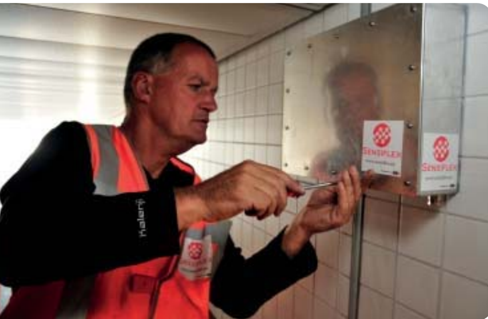
Figure 4.1.1. Nikhef technician Gerrit Brouwer installs a SensiQex RASNIK system in the Rotterdam Weena tunnel.
