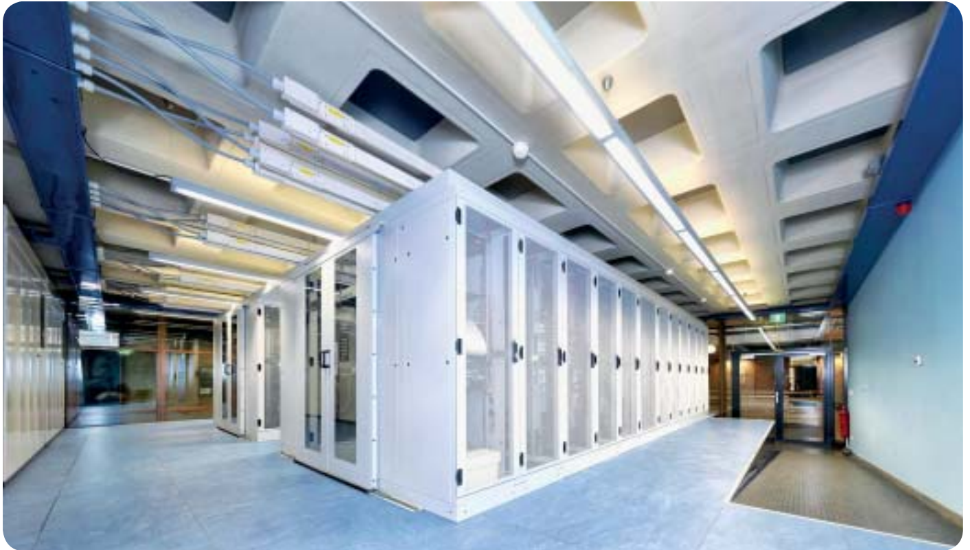
Figure 2.3.3.2: LHC Tier-1 machines in the new Nikhef data centre, commissioned in 2009.
