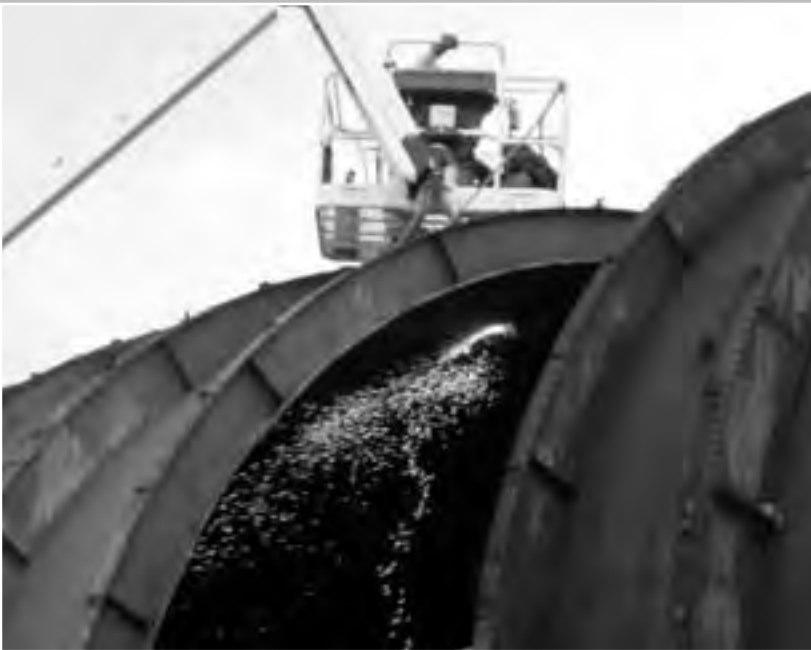
Image 285: A construction worker uses a torch to segment the inner shell. (NASA C-2008-04596)
