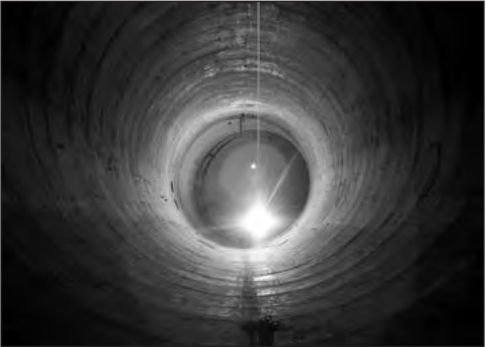
Image 291: A photographic survey of the AWT in April 2007 prior to its demolition. (NASA C-2007-00383)
