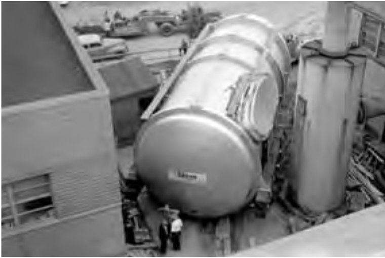
Image 128: The AWT modernization included the installation of a new exhaust gas cooler manufactured by Biggs Company, in Akron, Ohio. This photograph shows the large cooler being moved between the Shop and Office Building to the left and the Exhauster Building to the right. The cooler was installed below the tunnel's air scoop. A new 60-inch-diameter scoop was also installed. (NASA C-1951-28229)
