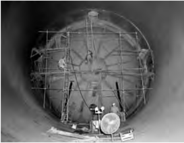
Image 182: Workers install a 31-foot bulkhead inside the southeast corner of the tunnel. The interior of the SPC was sandblasted and repainted with a double coat of aluminum paint that would not off-gas in a deep vacuum. 388 (NASA C-1961-58579)
