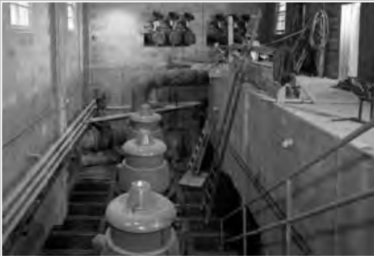
Image 129: A pump house was built underneath the northeast leg of the tunnel. This Circulating Water Pump House drew cooling water to be used by the new exhaust system. The pump house contained four Ingersoll Rand pumps, two 250-horsepower discharge pumps, and two 300-horsepower spray pumps. Another 75-horsepower spray pump was located in the northeast corner. These pumps drew and returned water from the Cooling Tower. (1951) (NASA C-2007-02591)
