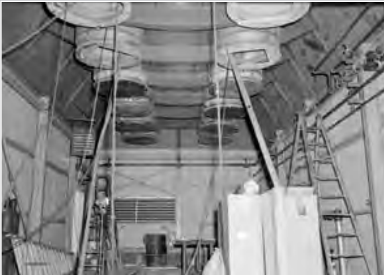
Image 185: Interior view of Vacuum Pump House being constructed below SPC No. 1. The portals for the 10 pending 32-inch-diameter oil-diffusion pumps can be seen in the ceiling of the pump house, which was directly underneath the chamber. (NASA C-1961-58582)
