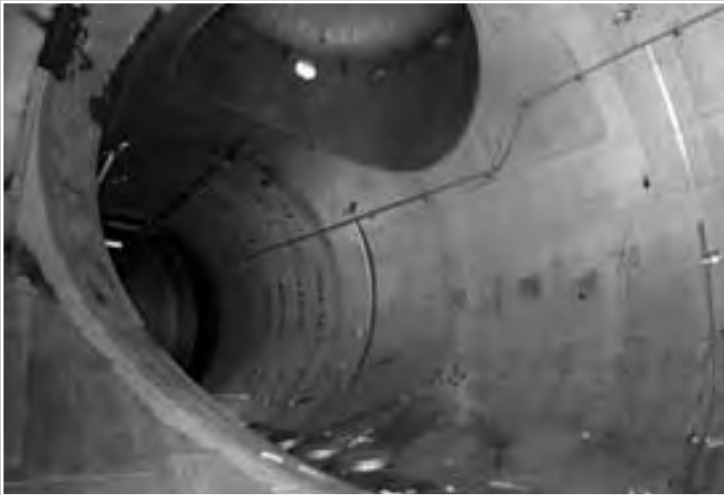
Image 272: Interior of SPC No. 1. Over the years, rain entered the open portals in the dome and collected on the chamber floor. This resulted in heavy rust damage along the bottom of the otherwise robust chamber. (NASA C-2005-01646)
