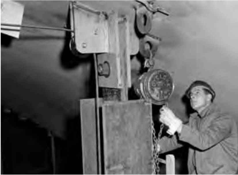
Image 238: A mechanic installs the new platform elevator in SPC No. 2 for a series of Centaur/OAO shroud tests. (NASA C-1965-00138)
