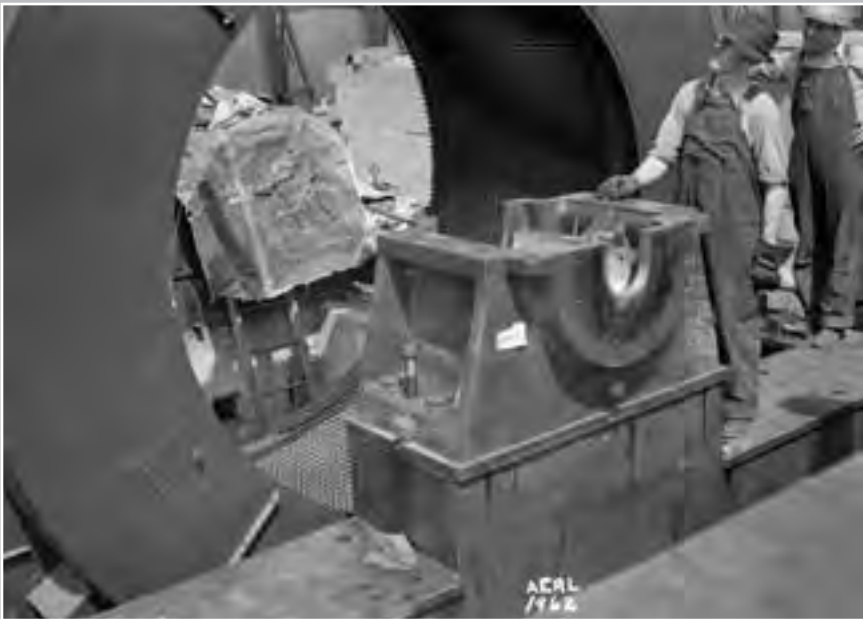
Image 32: During July 1943 the AWT's drive motor was installed in the northwest corner of the Exhauster Building. The motor, whose support frame is seen in this photograph, connected to the drive shaft that extended from the building, through the tunnel shell and into the AWT's fan assembly. The 18,000-horsepower General Electric Company induction motor was installed, and the corner of the building was built around it afterward. (1943) (NASA C-1943-01962)
