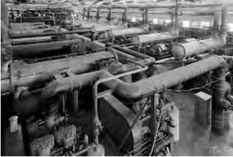
Image 95: The Carrier refrigeration equipment in the Refrigeration Building was activated to reduce the tunnel's air temperature to levels found at high altitudes. The building had its own control room and operators. It was the largest cooling system in the world when it was built and remains in use today. (NASA C-1944-06714)
