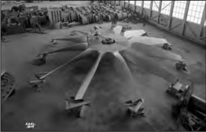
Image 26: NACA construction engineers Lou Hermann and Jack Aust assemble the AWT drive fan inside the hangar at the AERL. This 12-bladed, 31-foot-diameter spruce wood fan was designed at NACA Langley. John Breisch, a Langley technician with several years of wind tunnel installation experience, was brought up in July to supervise the fan assembly. He would return several weeks later to oversee the actual installation in the tunnel. 89 (NASA C-1943-01849)
