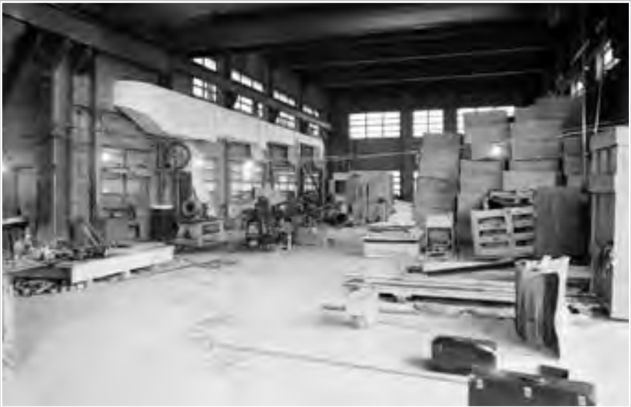
Image 34: Interior of the shop area inside the western wing of the AWT's Shop and Office Building as it was being constructed. (NASA C-1943-02186)
