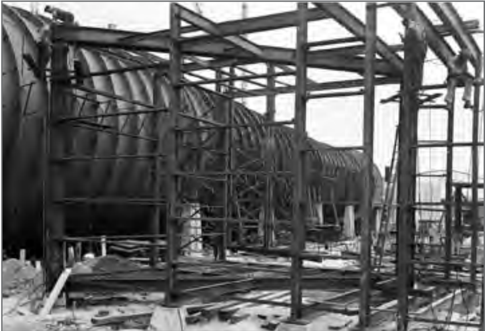
Image 16: The 1-inch-thick inner shell of the AWT is visible in this photograph of the facility being erected. The shell was made from a special steel alloy similar to current ASTM A710 Grade A3 steel plate. It was significantly stronger than normal carbon steel. (1943) (NASA C-2007-02314)
