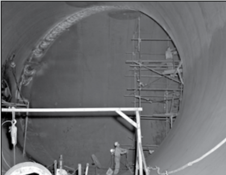
Image 179: Workers inside SPC No. 1 work at removing the former tunnel's turning vanes and cleaning up the chamber's interior. (NASA C-1961-58128)
