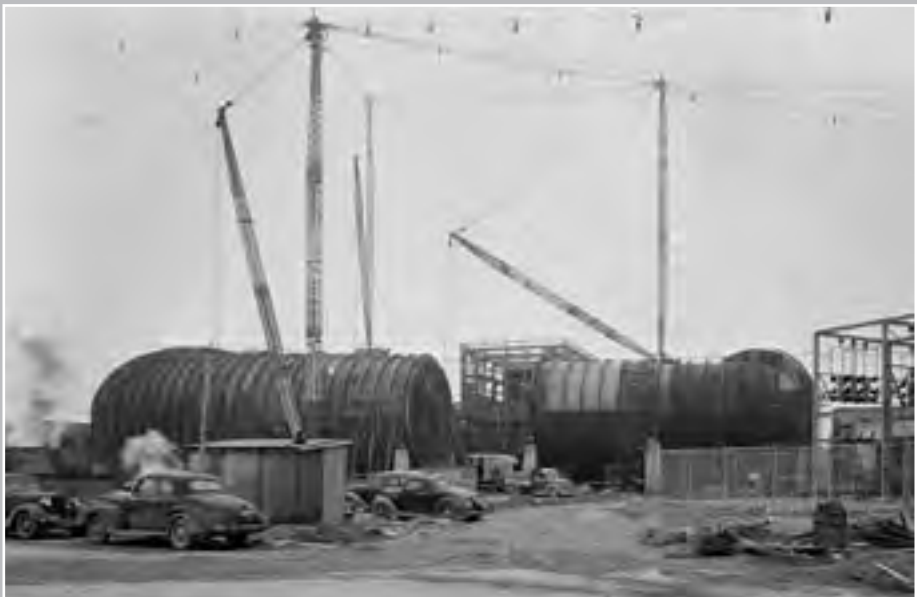
Image 30: Construction of the AWT with its test chamber visible in the center. Construction of the tunnel shell began in early 1943 and was completed in January 1944. In this photograph, the outer layer of the shell had yet to be installed (viewed from the south). (NASA C-1943-01521)
