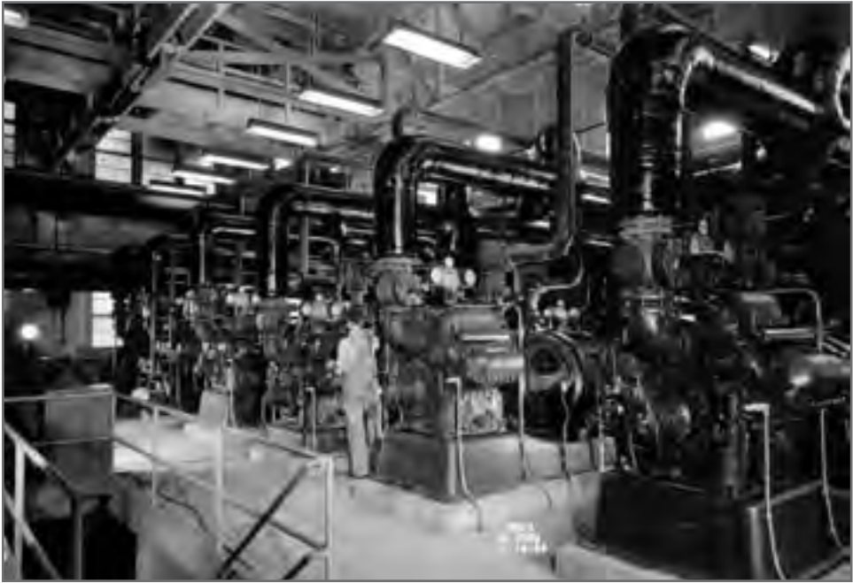
Image 18: Interior of the Refrigeration Building showing the 14 Carrier Corporation 1,500-horsepower centrifugal compressors that were the backbone of the AWT's complex cooling system. The system was used to cool the airflow in both the AWT and the Icing Research Tunnel. The building also contained York compressors, which were used to refrigerate the AWT's makeup air and provide institutional chilled water for the laboratory. (NASA C-1944-7456).
