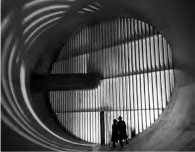
Image 99: Turning vanes were located in each corner to straighten the airflow and direct it around the tunnel's square corners. The fan's drive shaft can be seen penetrating this set of vanes. (NASA C-1944-03991)
