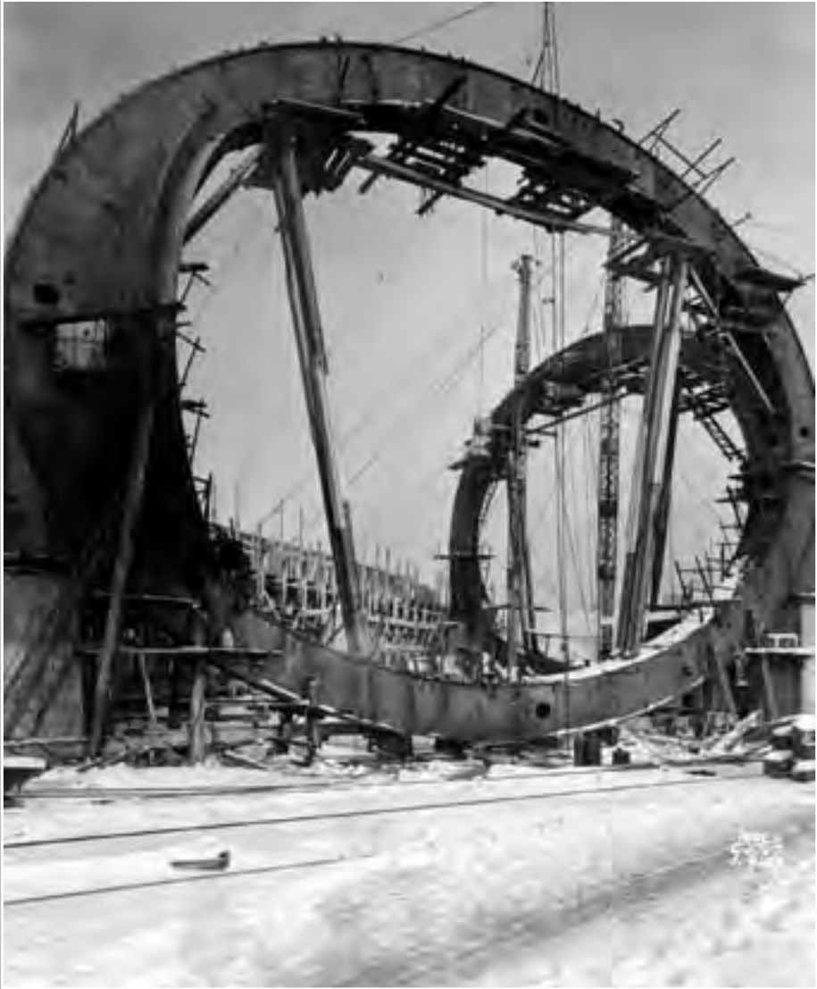
Image 28: Corner rings for the AWT are raised into place on 9 January 1943 during the early phases of the shell's construction. The Pittsburgh-Des Moines Steel Corporation constructed most of the enormous 263-foot-long, 120-foot-wide rectangular tunnel. The ring in the foreground had a 51-foot interior diameter. (9 Jan. 1943) (NASA C-1944-06707)
