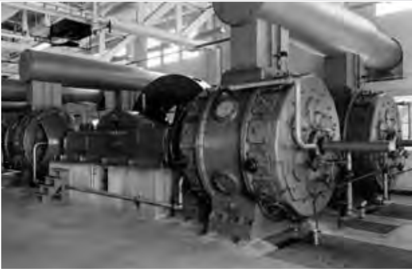
Image 96: The massive exhausters in the AWT Exhauster Building interconnected with the Engine Research Building's exhaust system and also, after 1951, to the Propulsion Systems Laboratory's exhaust system. Originally the tunnel's atmosphere could be reduced to simulate a pressure altitude of 50,000 feet. This was later improved to 100,000 feet. (NASA C-1944-06710)
