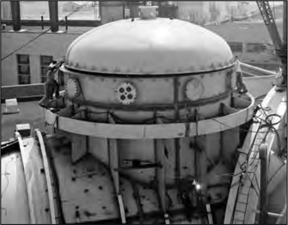
Image 191: An extension and dome are added to SPC No. 1 to accommodate a full-scale Centaur rocket. A crane lifts the dome's lid into place as a welder works below shoring up the supports. This photograph was taken in August 1963, almost a year after the facility was supposedly completed. (7 Aug. 1963) (NASA C-1963-65692)
