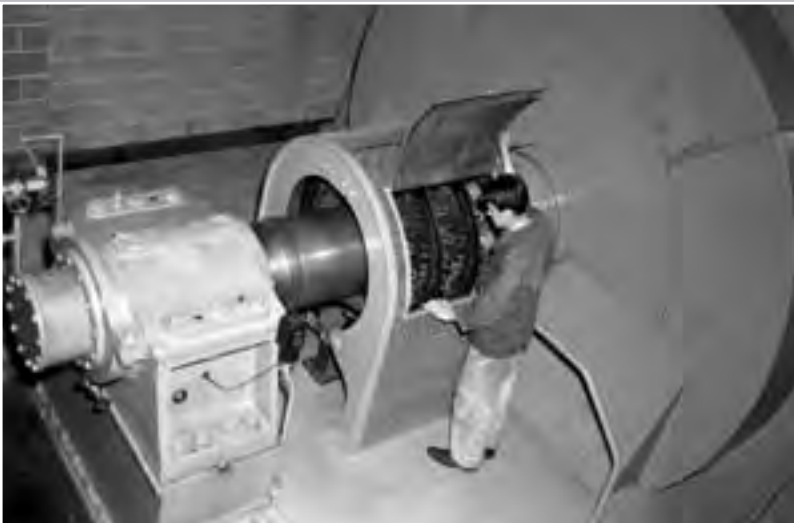
Image 98: An 18,000-horsepower General Electric induction motor was used to rotate the AWT fan assembly. The motor was housed in the third story of the Exhauster Building. Its drive shaft exited the building then penetrated the tunnel wall and coupled into the fan assembly. Two large generators on the first floor were activated first to supply power to the drive motor. (NASA C-1947-18325)
