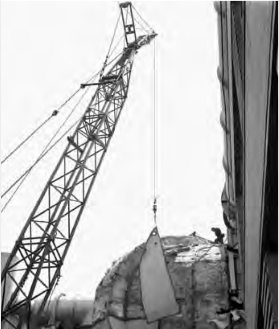
Image 181: The AWT's outer steel shell is removed so that the inner steel tunnel can be checked for leaks. The middle layer of insulation is visible. It was found that, in the push to complete the original tunnel construction during World War II, the seams were poorly welded. To create the vacuum chamber, NASA would have to reweld the entire east end of the tunnel. (NASA C-1961-57394)
