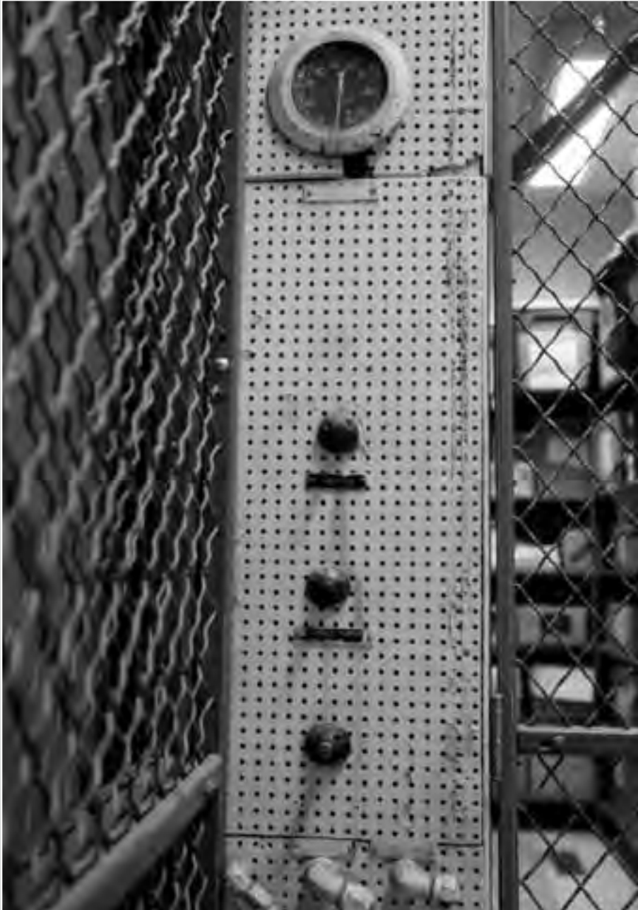
Image 273: This panel and the acoustical tile walls are the only remaining signs of the former AWT control room. The room was used to operate SPC No. 2 tests in the 1960s and 1970s, but the control panels and measurement equipment were removed over the years. The space is now used as a storage room. (NASA C-2007-00398)
