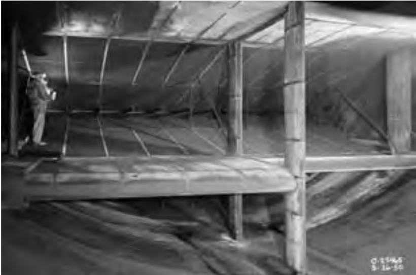
Image 100: The airflow passed through a bank of accordion-shaped cooling coils specially designed to reduce the AWT's temperature to -47^{\circ}\text{F} . As the air passed through the banks of coils, heat was transferred to liquid Freon in the coils and carried away. (NASA C-1950-25465)
