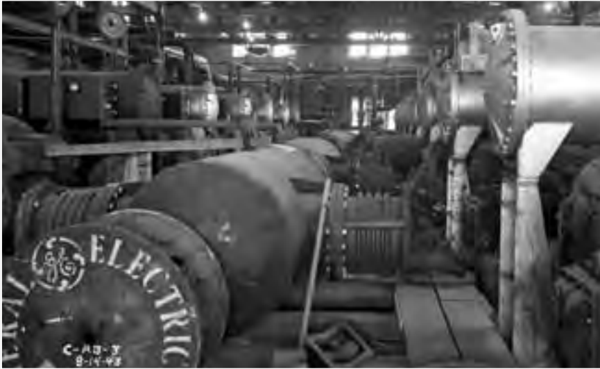
Image 31: Interior of the Refrigeration Building with the flash cooler in the center of the photograph. The flash cooler would be connected to the distributing headers and the Carrier compressors along both the left and right. (NASA C-2007-02318)
