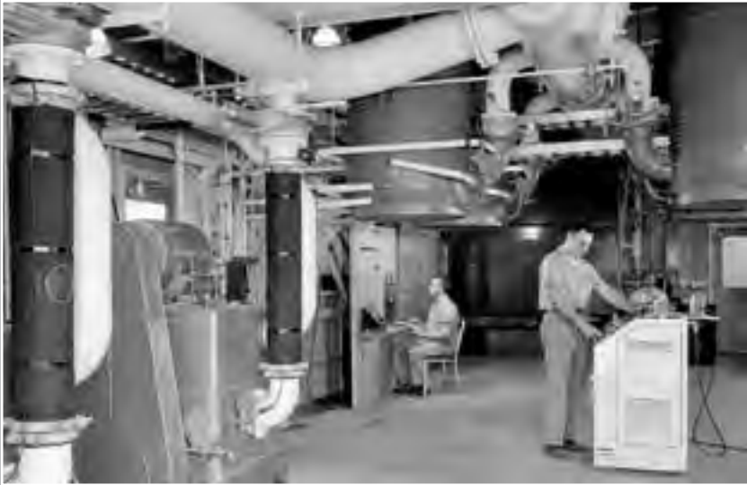
Image 215: The Vacuum Pump House contained the two Stokes piston pumps, which could remove 12.5 cubic feet of air per second during the roughing stage; a Roots rotary positive displacement pump, which could then remove 500 cubic feet per second; and ten 32-inch-diameter oil-diffusion pumps, which could remove 17,650 cubic feet of air per second. 459,460 (NASA G-1962-60342)
