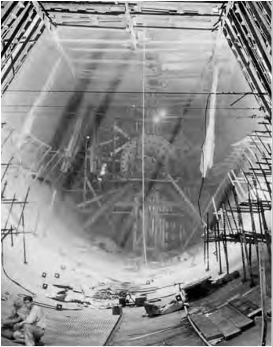
Image 35: Interior of the AWT's southern leg during construction. The propeller bearing supports are in place, and the bearing box propeller hub and drive shaft are being installed at the far end. (1943) (NASA C-1944-04710)
