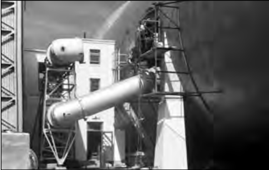
Image 79: Construction of the Small Supersonic Tunnel behind the AWT in June 1945. This would be the lab's first supersonic tunnel. Eventually the building would house three small supersonic tunnels, referred to as the "stack tunnels" because of the vertical alignment. The two other tunnels were added to this structure in 1949 and 1951. (NASA C-1945-10764)
