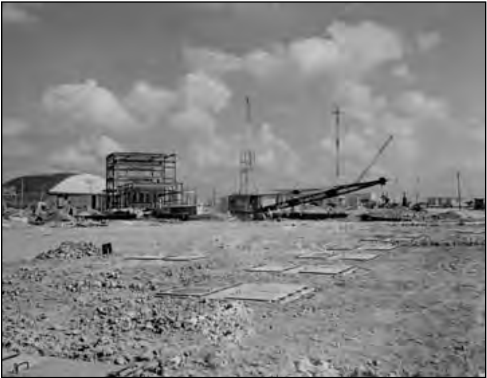
Image 21: This photograph from late spring 1942 shows the construction of the AWT's Shop and Office Building. The tunnel's steel and concrete piers can be seen behind the crane. The Sam W. Emerson Company would complete this task by late December. The hangar, the first AERL building completed, is in the background. Retiree Frank Holt recalled that during this period the surveyors were "out everyday in their high-top boots with their tripods and scopes" in the mud laying out the new lab. 76 (1942) (NASA C-2007-02306).
