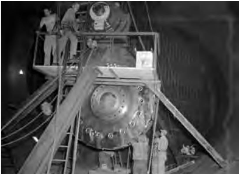
Image 127: Workers install a large hub as part of a large overall upgrade of the AWT. The blades, hub, and fairings for the drive fan were replaced. The new fairings were roughly twice the original size. (NASA C-1951-28286)
