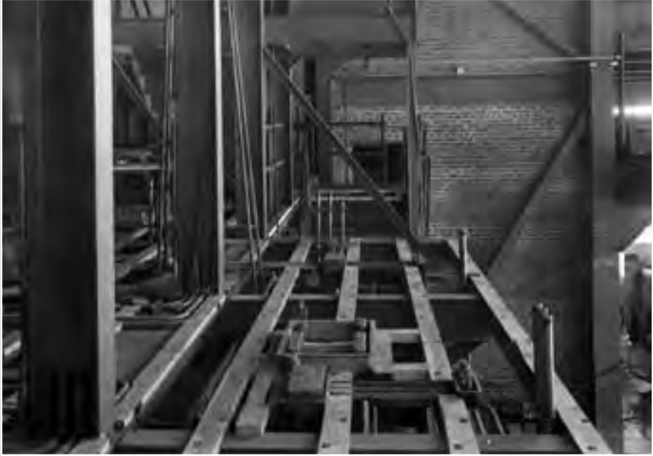
Image 33: Construction of the viewing platform in the AWT's Shop and Office Building. The platform is in the rear of the high bay. The shop can be seen below to the right. The lower half of the tunnel's test section, out of view to the left in this photograph, was sunken below the platform so that the test articles were near the floor level. (NASA C-2007-02298)
