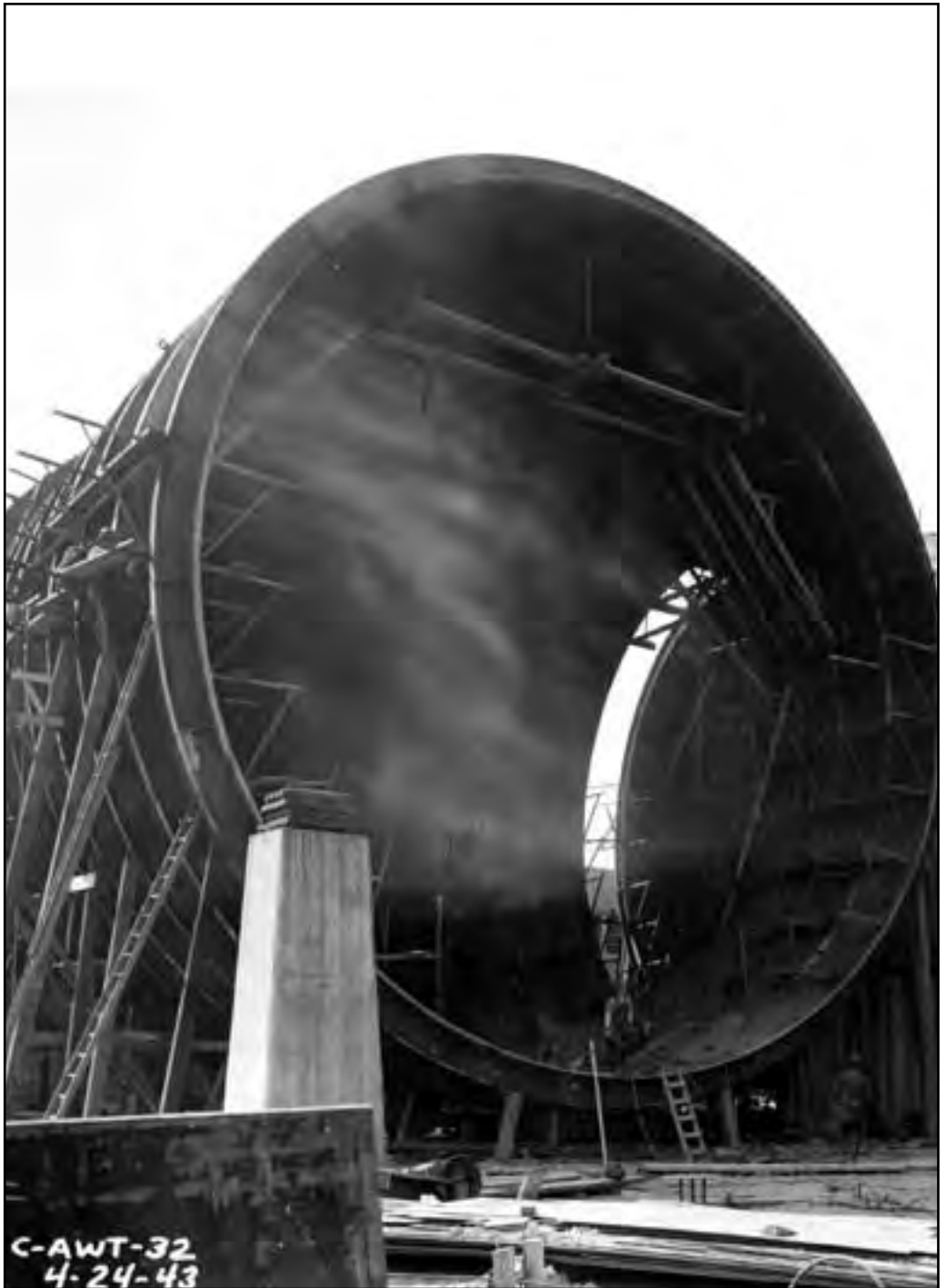
Image 14: The Altitude Wind Tunnel as its shell is constructed by the Pittsburgh-Des Moines Steel Company in April 1943. (NASA C-2008-00817)
