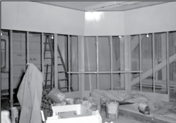
Image 180: Construction of a new control room for SPC No. 1 beneath the tunnel's test section. (28 Nov. 1961) (NASA G-1961-58575)
