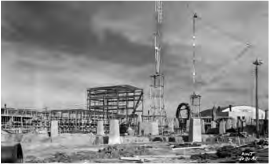
Image 29: Steel framework for the Shop and Office Building is at the left, with one of the tunnel's corner rings standing vertically. The completed aircraft hangar is in the background, and the tunnel's foundations are in the foreground (viewed from the southwest). (1942) (NASA C-2007-02294)
