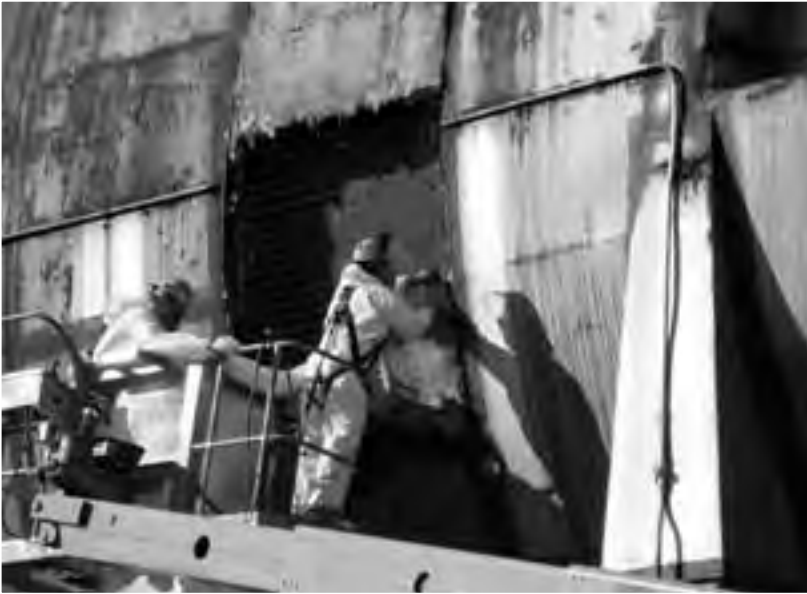
Image 284: The insulation and steel mesh are removed from between the shells. (NASA C-2008-04591)
