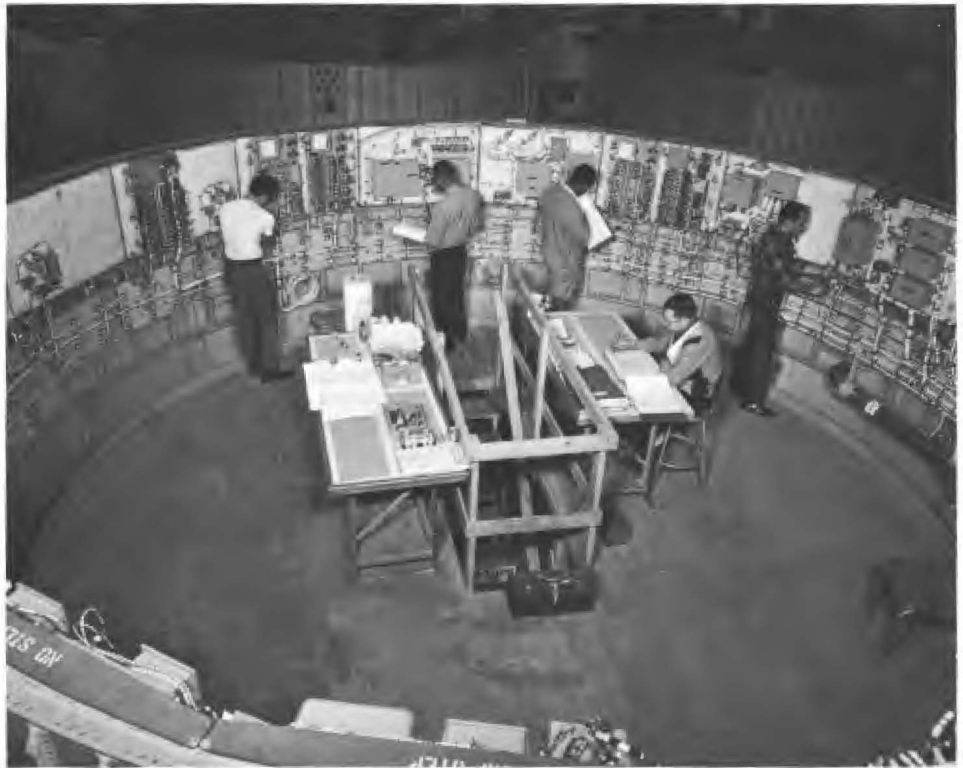
Douglas engineers are shown installing the electrical system in the forward area of the S-IVB stage.
