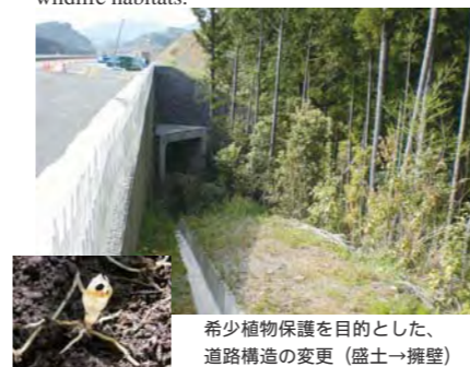
Design Change for the Purpose of Rare Plants Protection (Embankment Retaining Wall)
