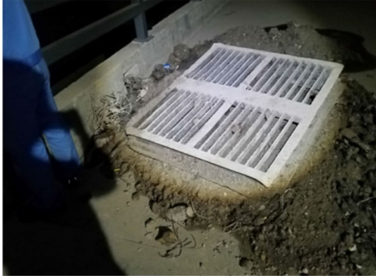
Figure 11 Stainless wastewater screen
