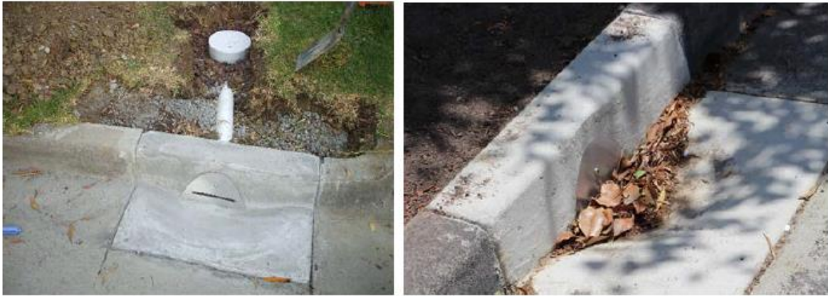
Figure 5-7 Photographs of installed TreeNet inlet system. Source: 2018 ZAM-WSUD Handbook.
