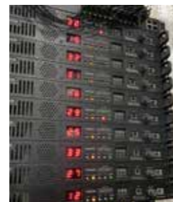
The status of communication is indicated by numbers and lamp color
