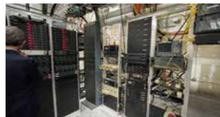
A repeater installed in the hotel's server room
