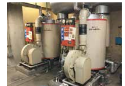
Fossil fuel boiler before decommissioning (JVCKENWOOD Nagano Corporation)
