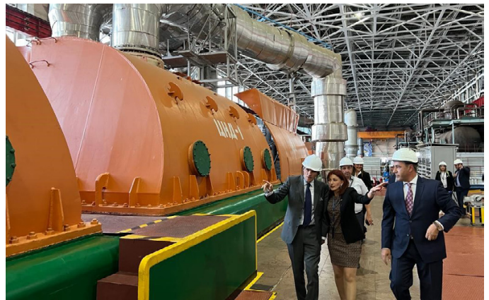
In 2022 IAEA DG Rafael Mariano Grossi visited the Metsamor Nuclear Power Plant in Armenia (Photo: D. Candara)
