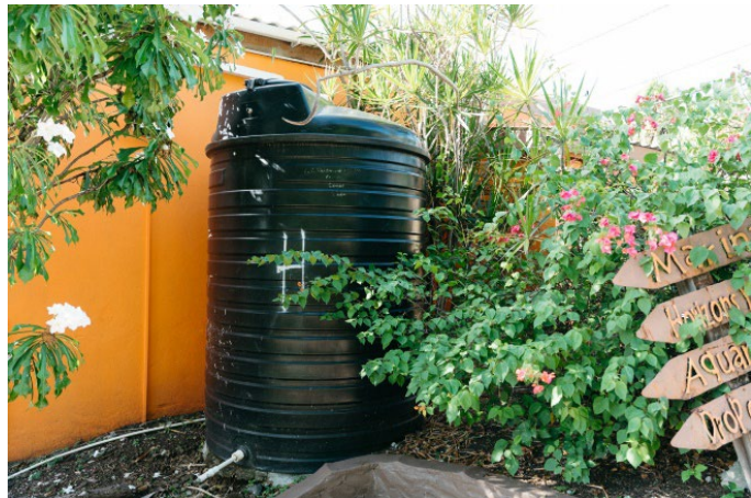
Rainwater harvesting system installed at True Blue Bay resort. Photo: Communications Unit/GIZ
