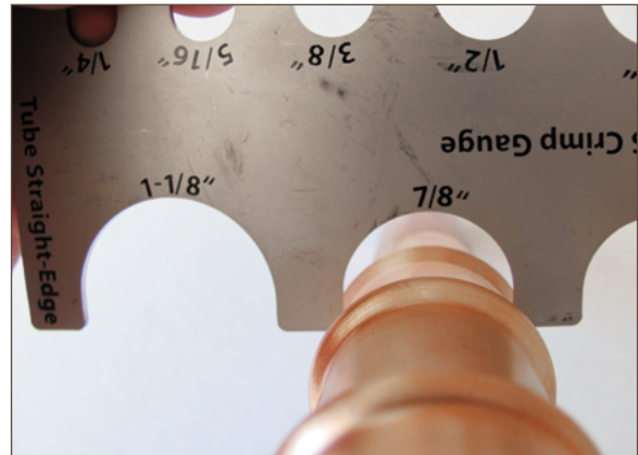
Figure 11.21. Un-crimped or improperly crimped fitting
