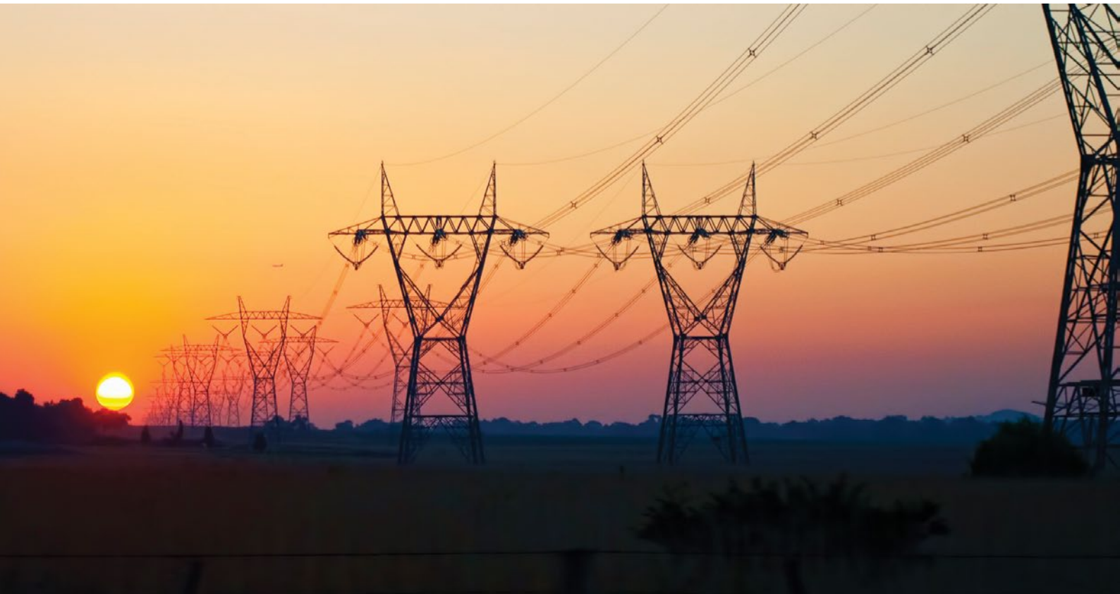
Figure 6: Power pylons in southeast Australia – climate change is worsening extreme weather including heatwaves and is increasing the vulnerability of energy systems to blackouts.
