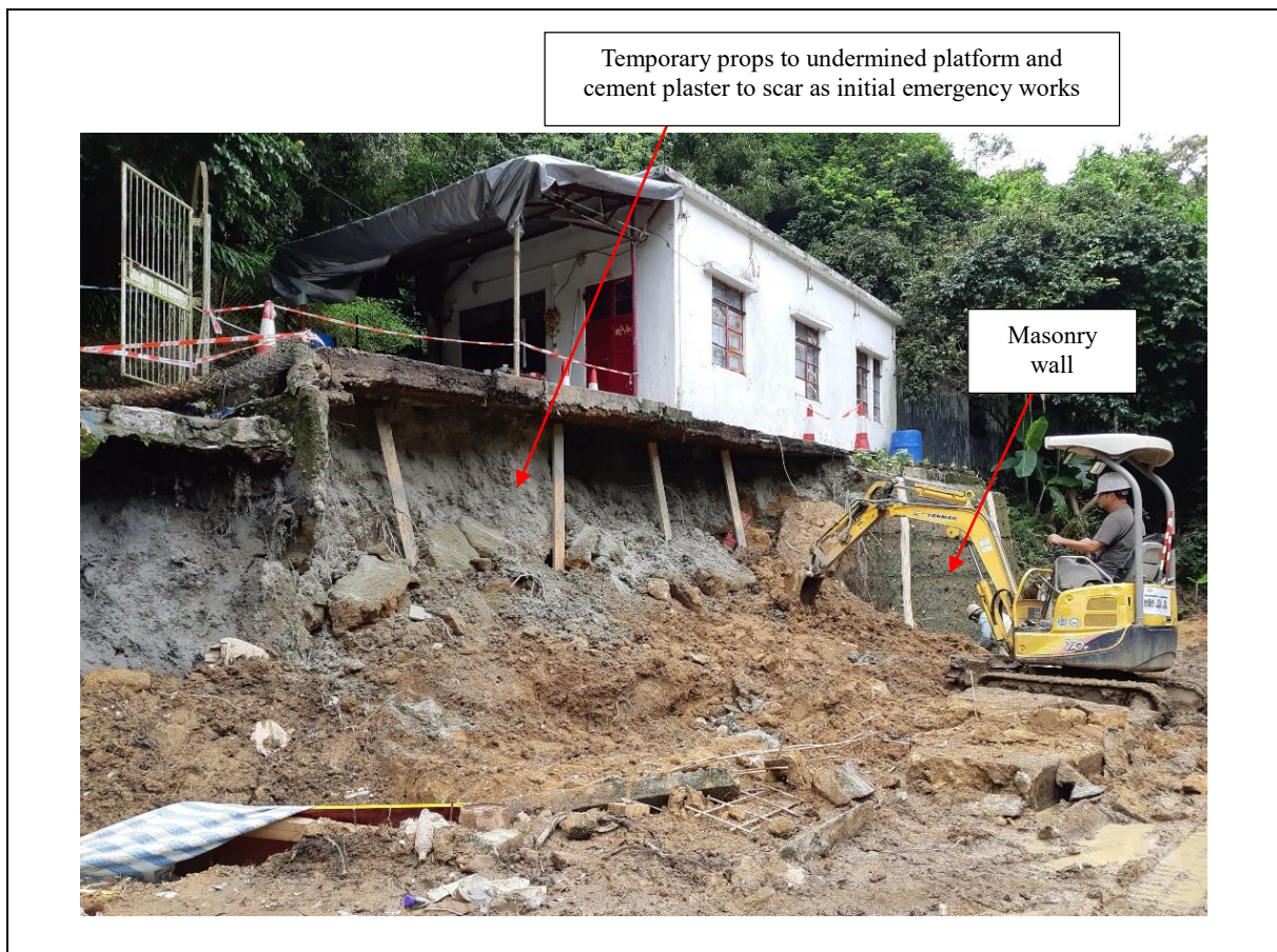
Figure 4.1 View of the 6 June 2020 Landslide on a Retaining Wall at South of No. 5 Tung Hang Mei, Mui Wo (Incident No. 2020/06/2637)
