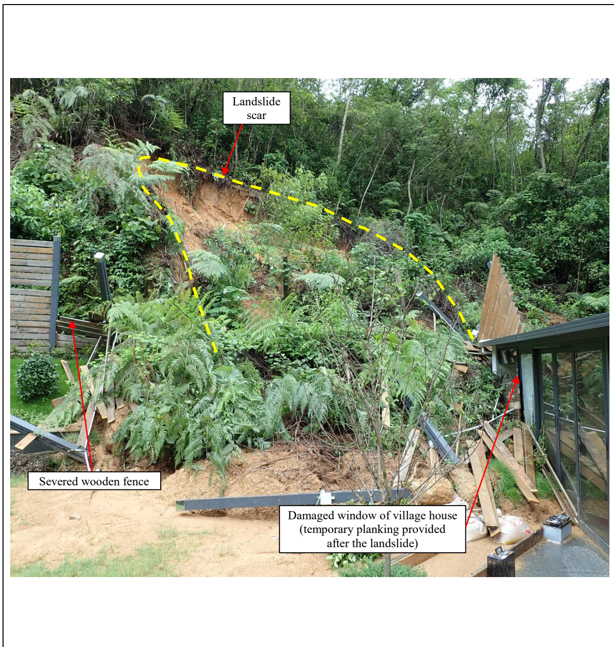
Figure 4.2 View of the 7 June 2020 Landslide on the Natural Hillside behind House No. 292, Lung Mei Village, Tai Po (Incident No. 2020/06/2663)
