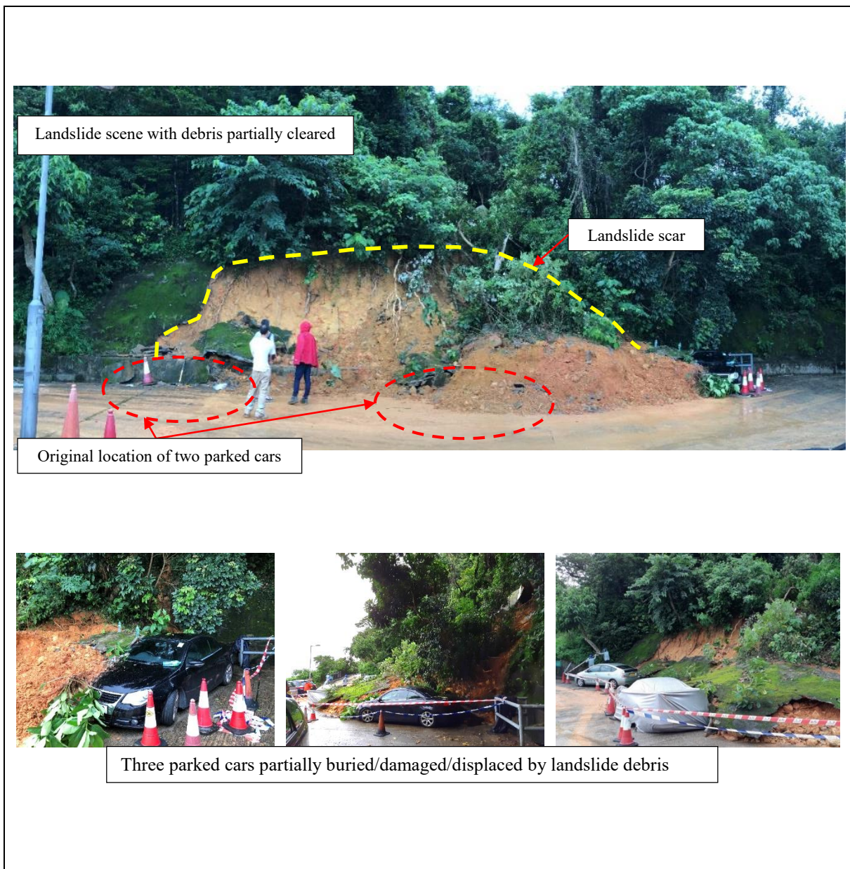
Figure 4.3 Views of the 6 June 2020 Landslide on a Soil Cut Slope at an Open Carpark at Shan Liu Ha Road, Sai Kung (Incident No. 2020/06/2631)
