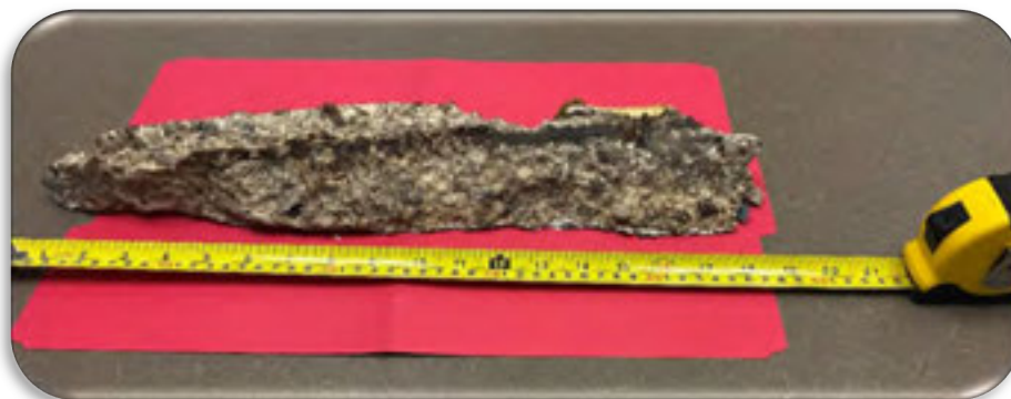
Figure 2 - Chunk of Concrete that Fell off Structure
