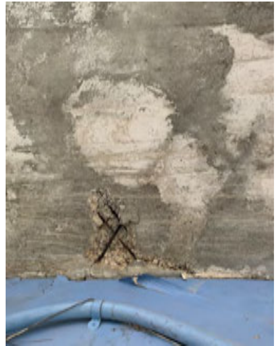
Photo 7. Severe concrete spalling and severely corroded steel reinforcing at roof line. Blue is interior wall.
