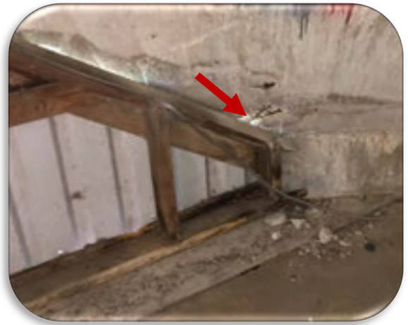
Figure 5 - Popout/Spall exposing reinforcing steel
