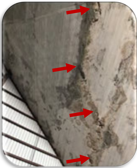
Figure 4 - Additional popout/spalls exposing steel reinforcement
