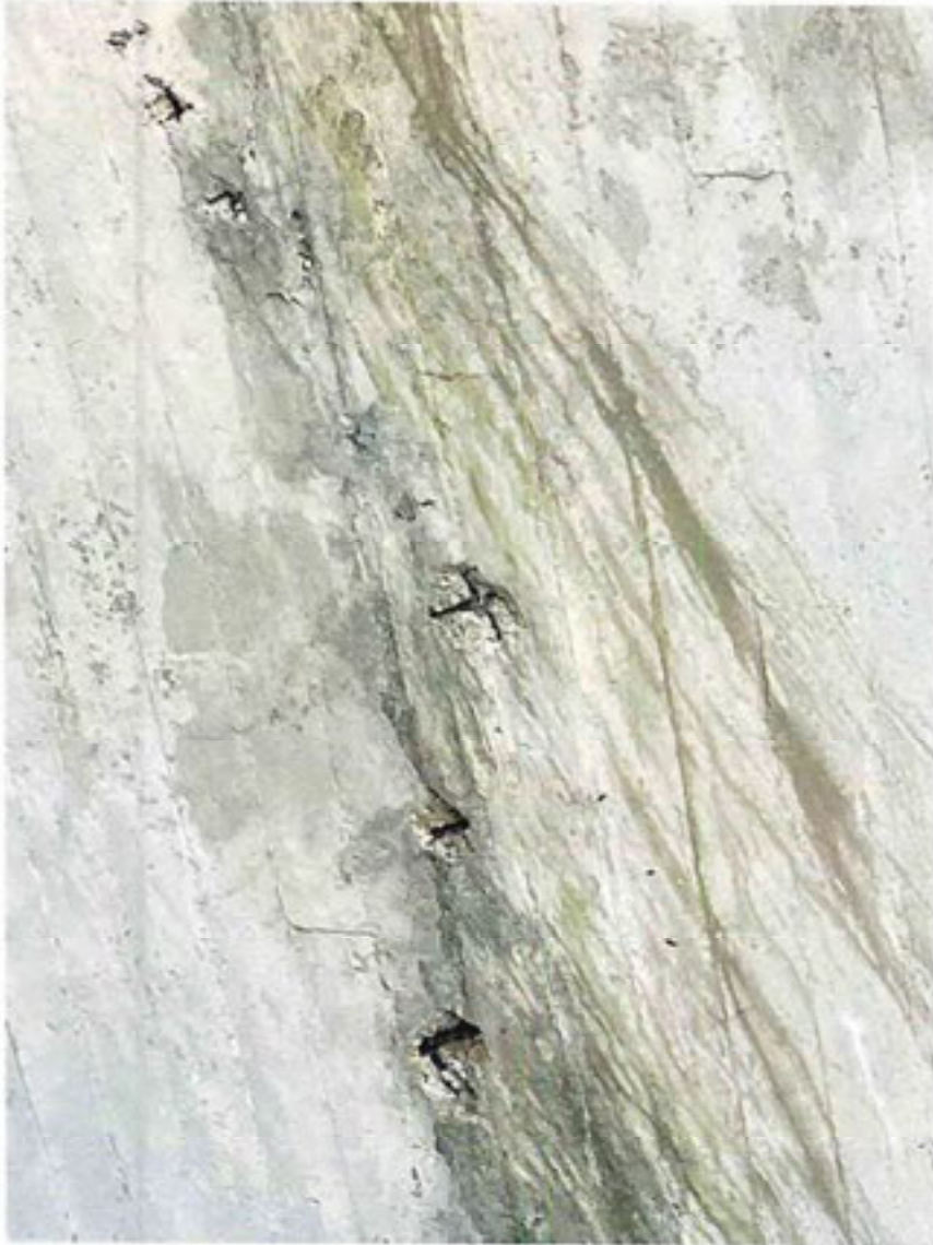
View of deteriorating concrete side walls within the East GA Hangar No. 1.
