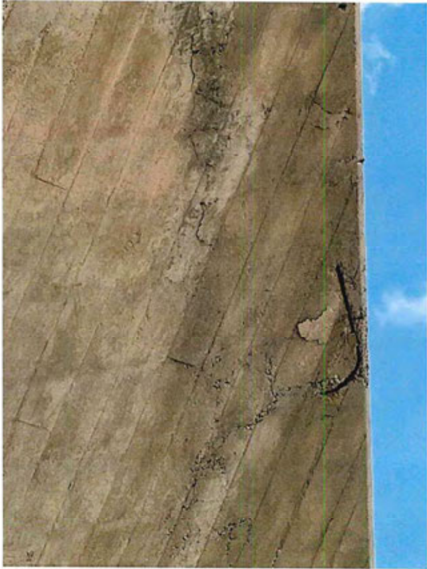
View of concrete roofing along east edge of East GA Hangar No. 1.
