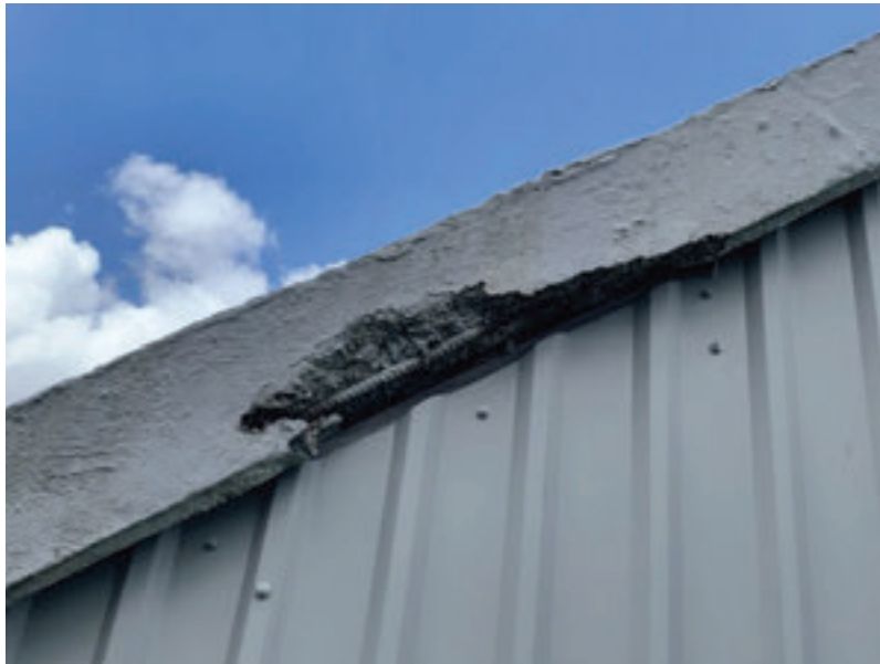
Figure 7: Severe concrete spalling and exposed unprotected steel reinforcing at structural support.
