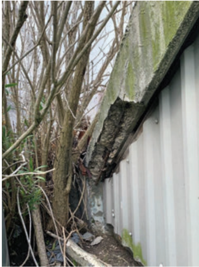
Figure 6: Severe concrete spalling and corroded steel reinforcing at existing structural support.
