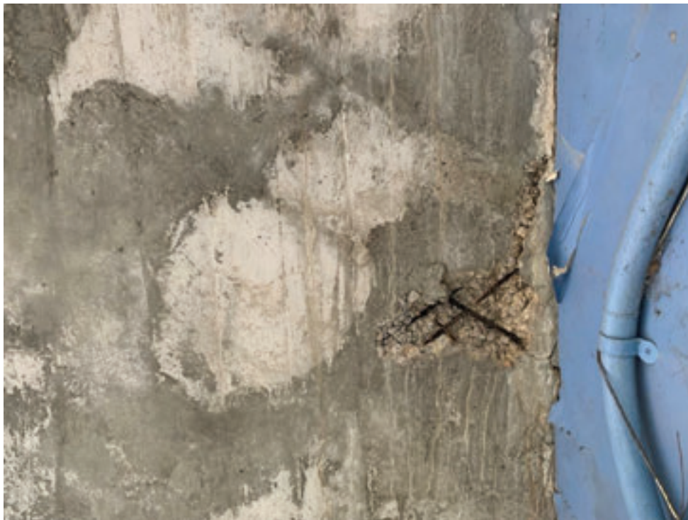
Figure 3: Spalling concrete and severely corroded steel reinforcing at existing roof.
