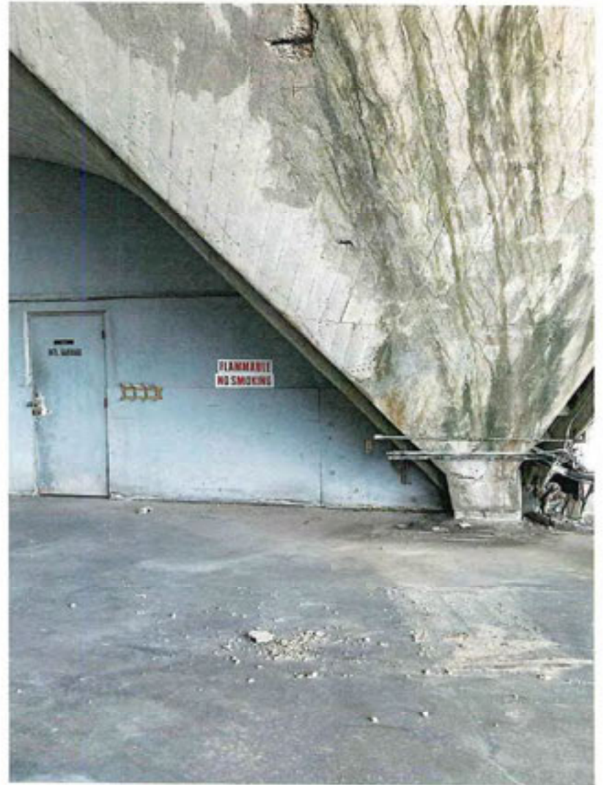
View of deteriorating concrete side walls within the East GA Hangar No. 1.
