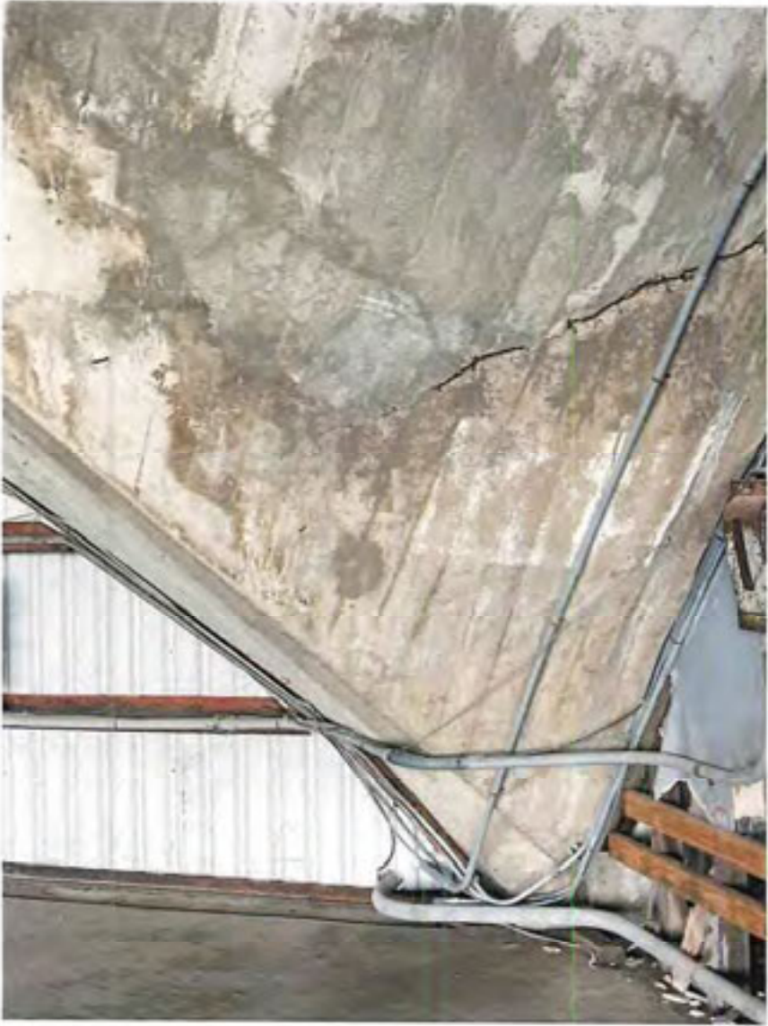
View of large crack in concrete side wall within the East GA Hangar No. 1.
