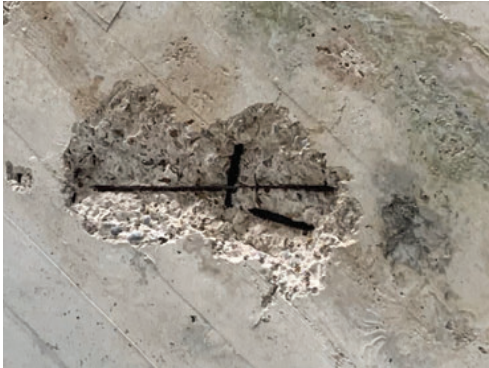
Figure 2: Spalling concrete and severely corroded steel reinforcing at existing roof.
