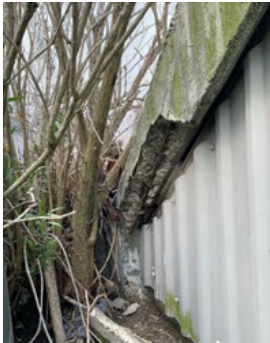
Photo 6. Severe concrete spalling and corroded steel reinforcing at existing support.
