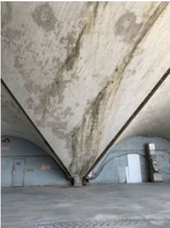
Photo 2. Severe concrete spalling and corroded steel reinforcing at existing primary structural support.
