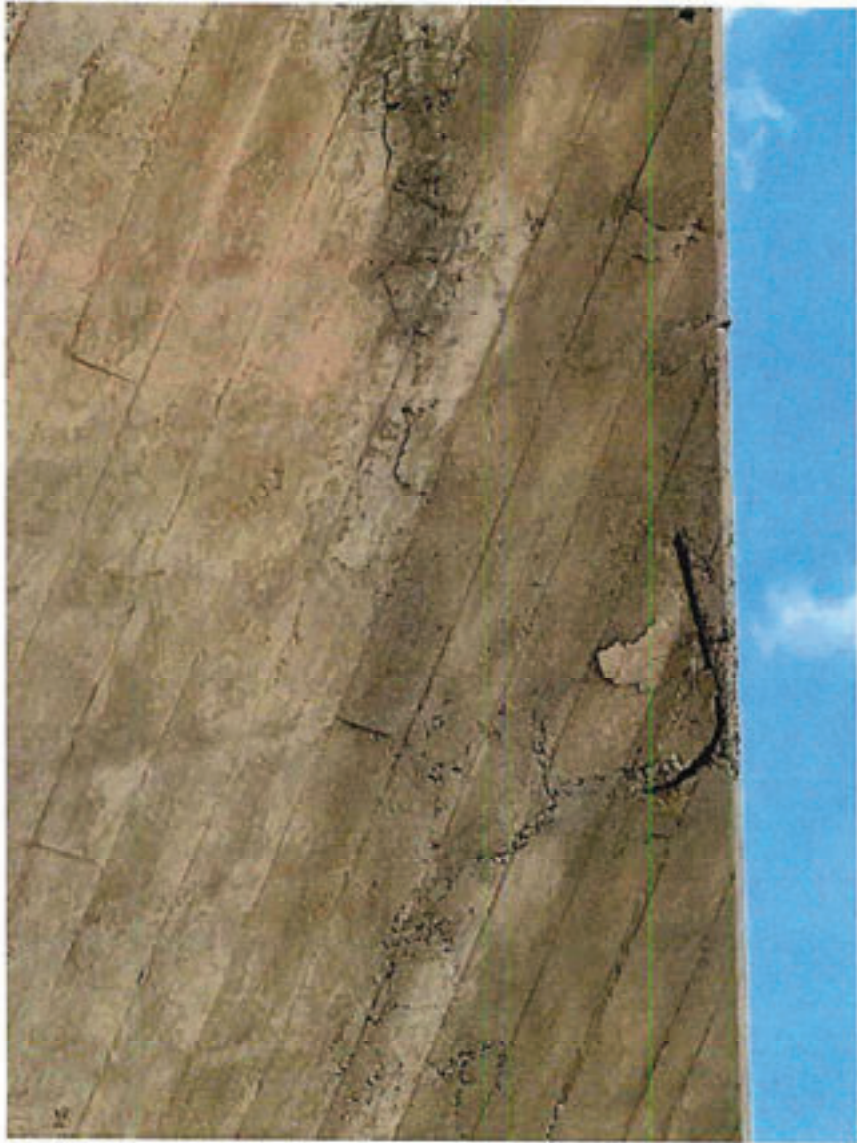
View of concrete roofing along east edge of East GA Hangar No. 1.
