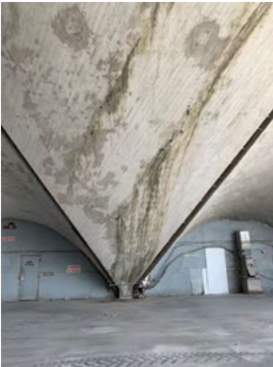
Photo 2. Severe concrete spalling and corroded steel reinforcing at existing primary structural support.
