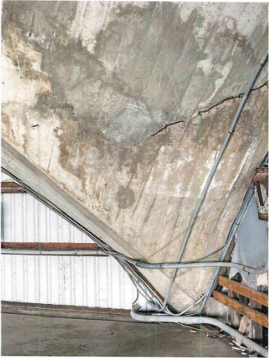
View of large crack in concrete side wall within the East GA Hangar No. 1.
