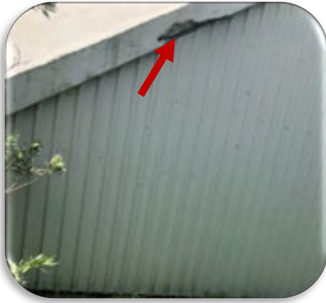
Figure 7 - Spall on concrete eave exposing steel reinforcement
