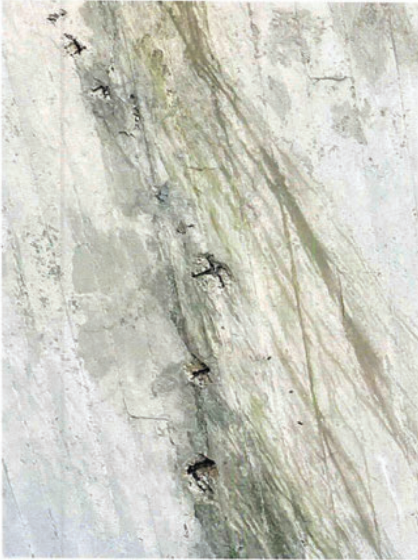
View of deteriorating concrete side walls within the East GA Hangar No. 1.
