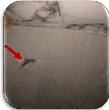
Figure 8 - Popout/Spall in finished office area exposing steel reinforcing
