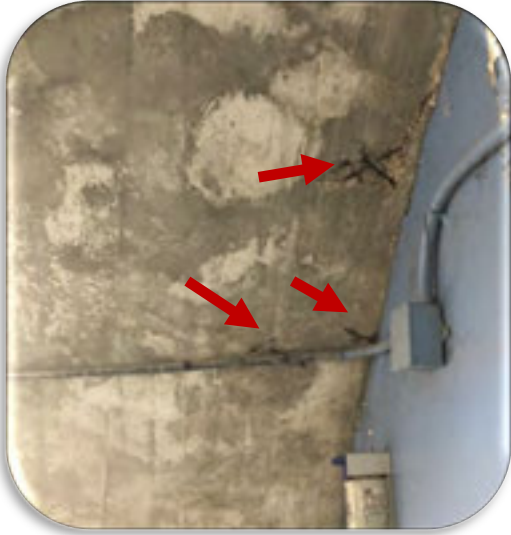
Figure 3 - Interior view of the hangar ceiling, note popout/spall exposing steel reinforcement.
