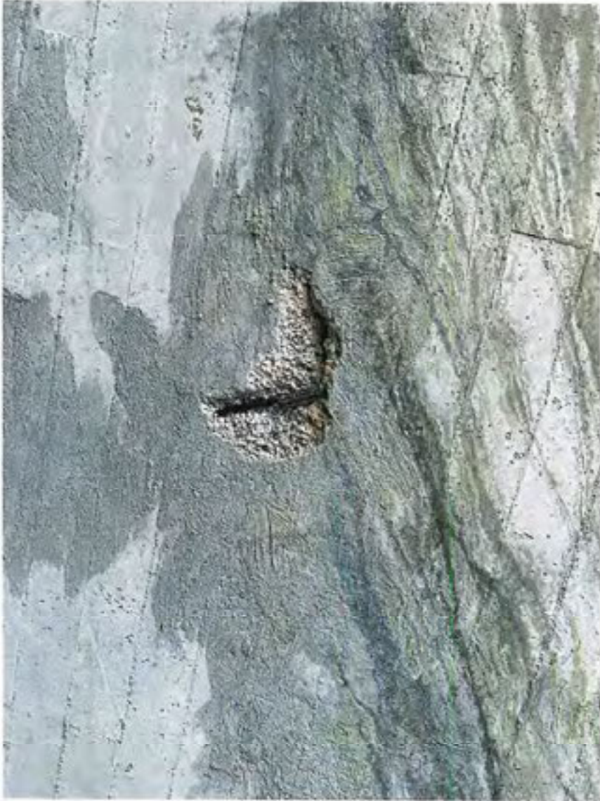
View of deteriorating concrete within the East GA Hangar No. 1.
