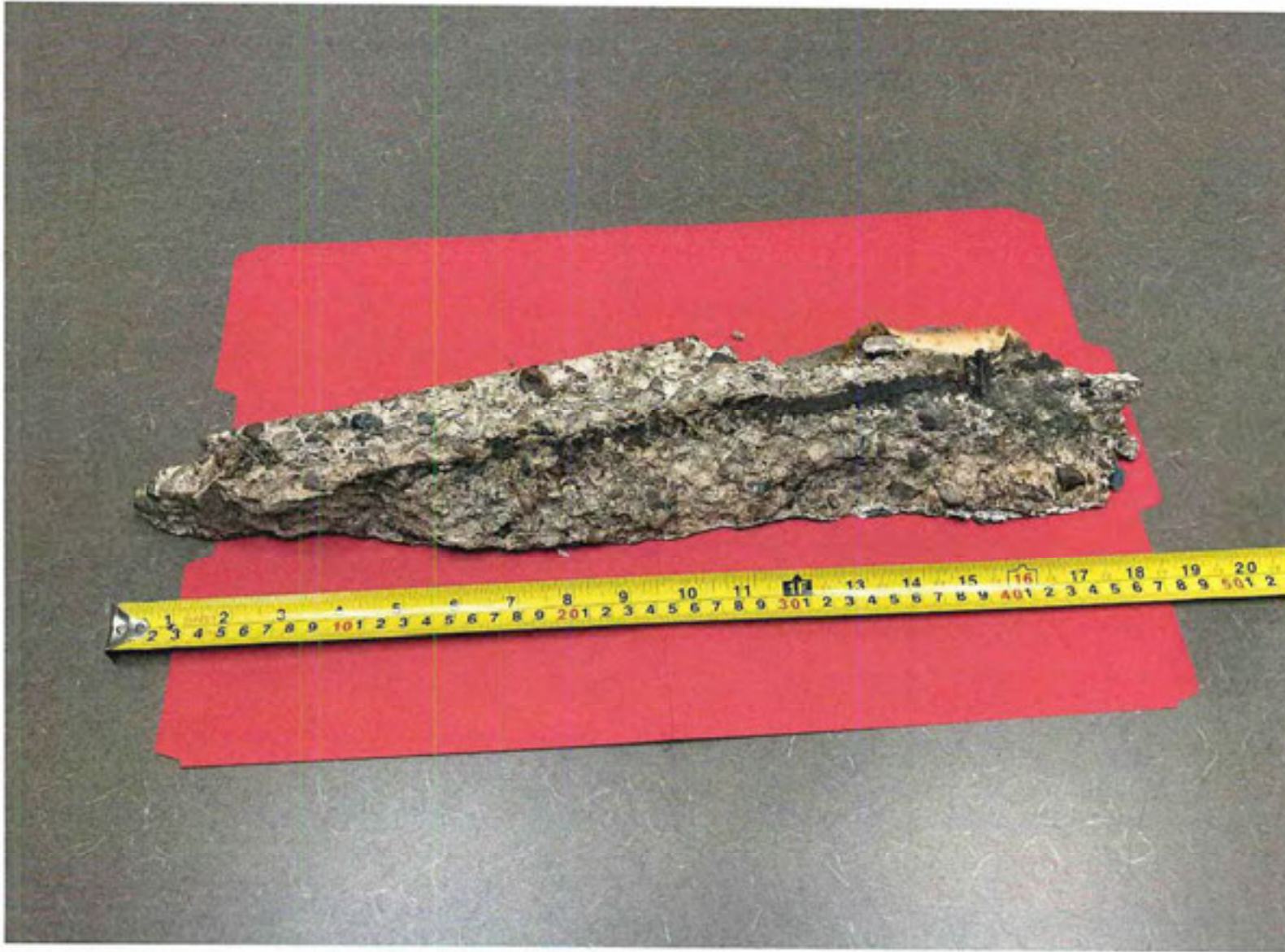
Large shard of concrete that has fallen from the East GA Hangar No. 1 structure.
