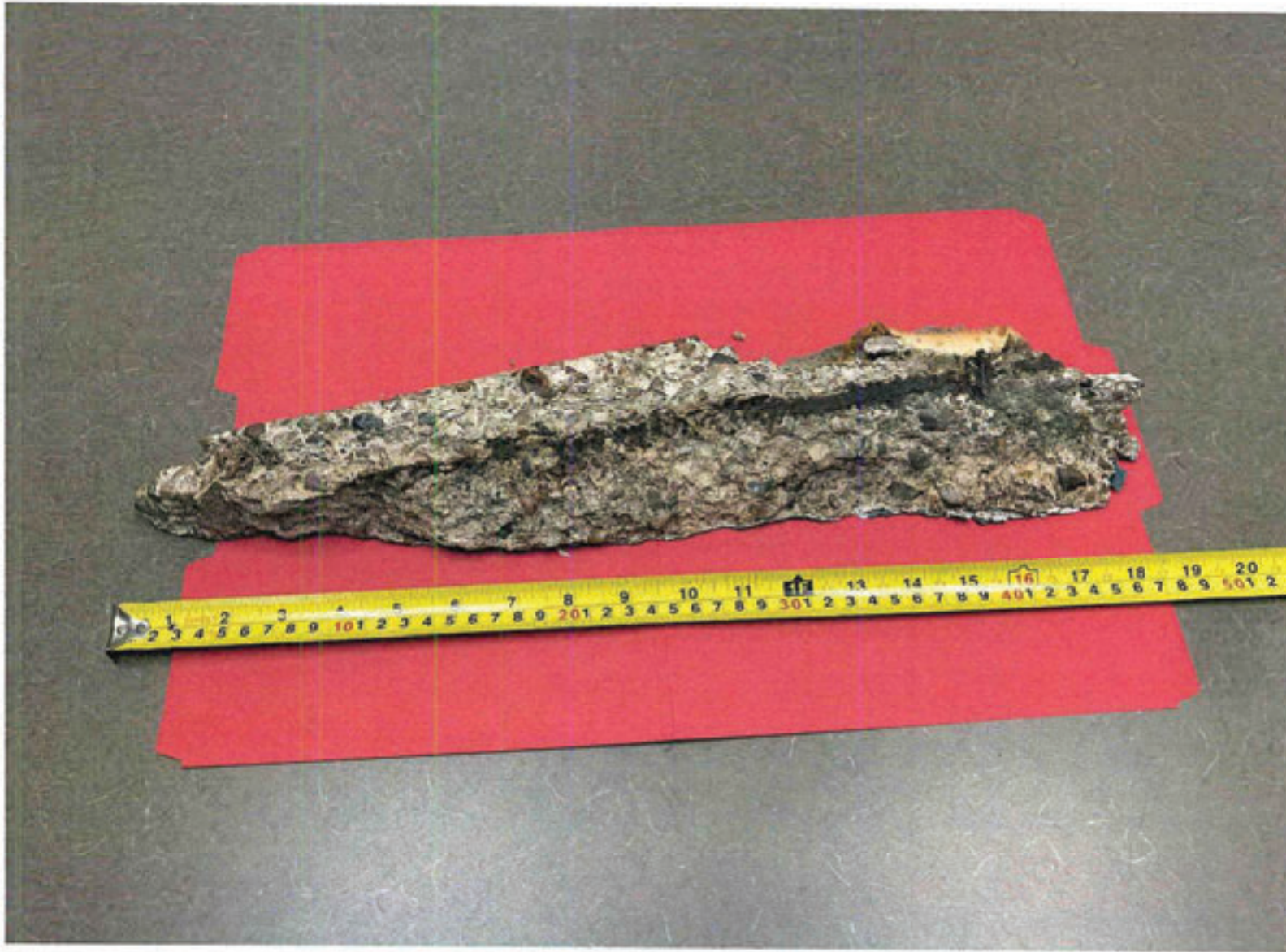
Large shard of concrete that has fallen from the East GA Hangar No. 1 structure.
