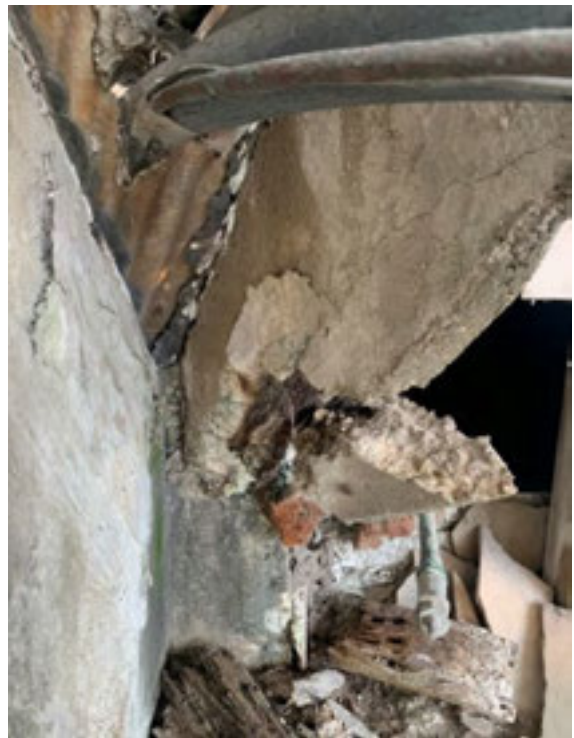
Photo 3. Sever concrete spalling and corroded steel reinforcing at existing primary structural support.
