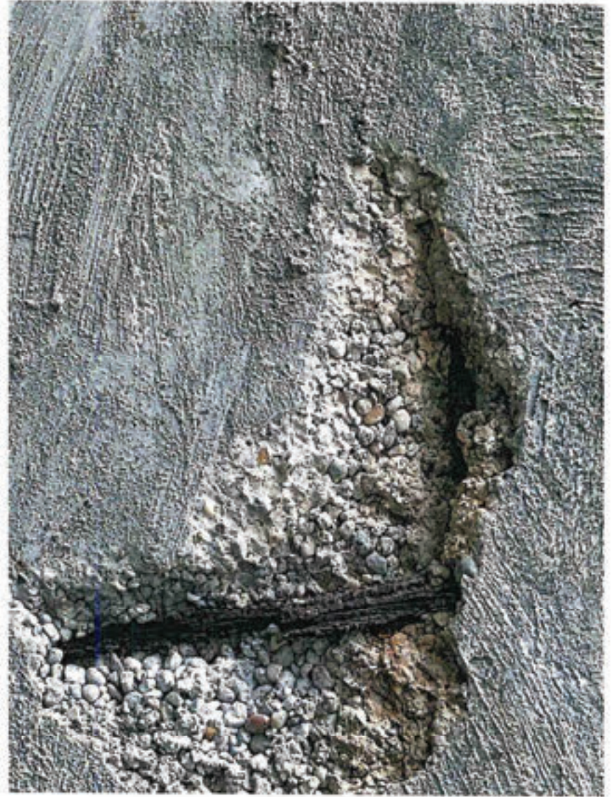
View of deteriorating concrete within the East GA Hangar No. 1.
