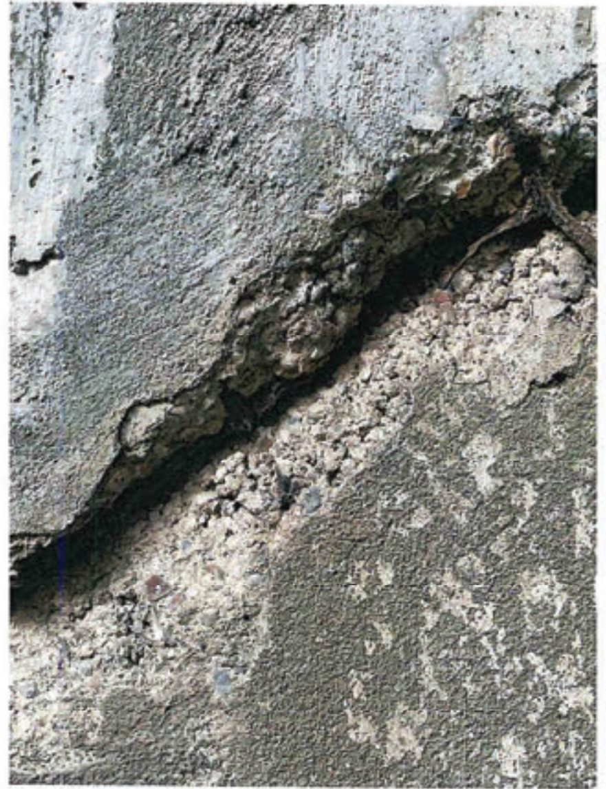
View of large crack in concrete side wall within the East GA Hangar No. 1.
