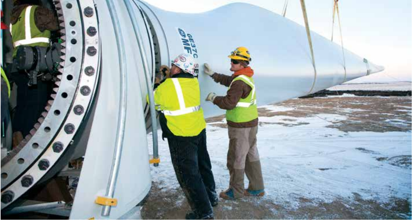
An additional 169.5 megawatts of wind resources were energized in North Dakota in 2009, of which 120 megawatts were from the first large-scale wind project built and owned by a Basin Electric subsidiary. The contractor for PrairieWinds ND 1, RMT, prepares a turbine blade for connection to the hub. The three-bladed rotor is lifted by crane to the top of the tower for connection to the shaft.
