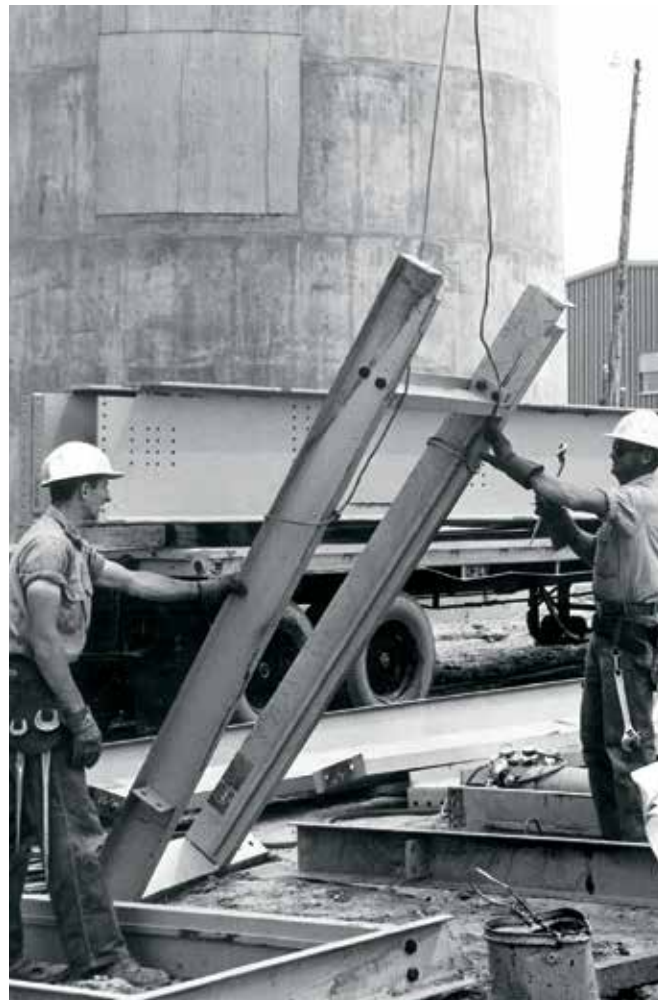
Workers prepare steel framework to be lifted to an area under construction of Leland Olds Station Unit 1.
