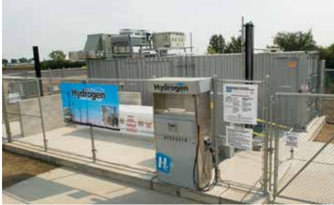
Through a federal grant and partnering with other cooperatives and researchers at two North Dakota universities, Basin Electric initiated a $2-million project to create hydrogen from the electricity produced by wind turbines.
