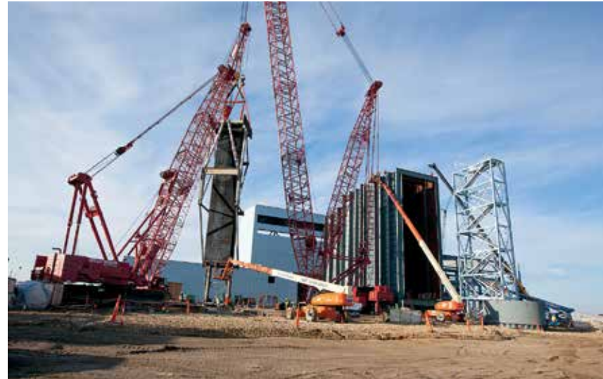
Boldt Construction places one of 14 70-foot-long heat recovery steam generator (HRSG) modules in April 2011 at the Deer Creek Station. The combined-cycle plant will have a gas turbine spinning one generator. Then the gas turbine’s hot exhaust is captured and sent through the HRSG modules to heat water for the steam turbine, which spins another generator.
