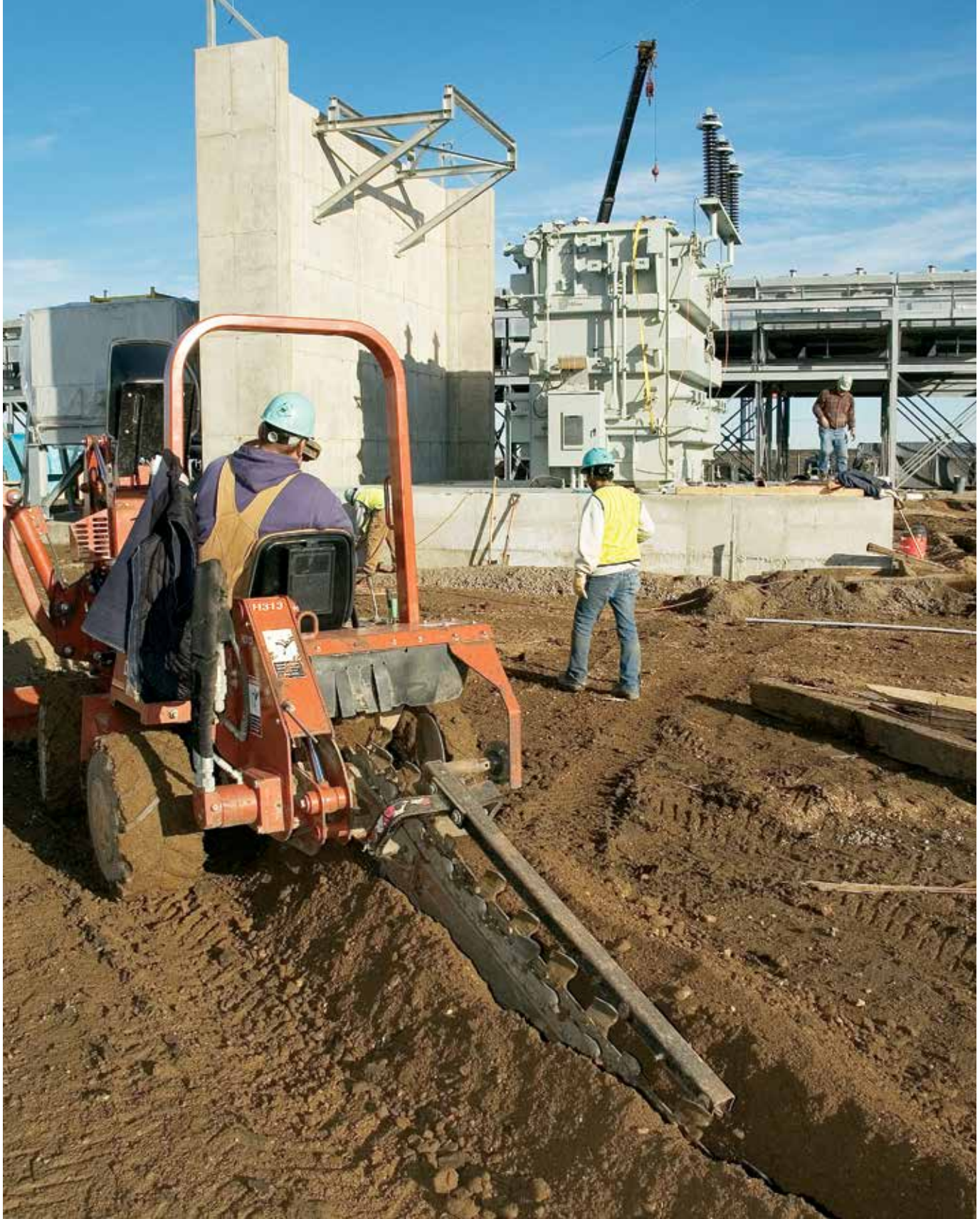
Construction work on Groton Generation Station Unit 1 shows the generator step-up transformer on the concrete foundation. A blast wall to the left will protect the turbine-generator to be placed on the other side in the event of a transformer fire or explosion.
