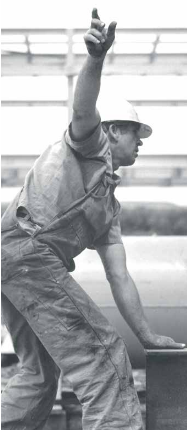
An unidentified worker signals a crane operator during construction of Unit 1 of the Leland Olds Station.
