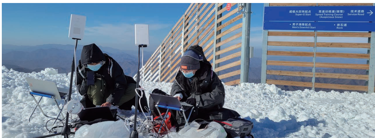
A Huawei team performs network maintenance and testing 2,000 meters above sea level on top of a mountain in Beijing, China to ensure the quality of high-definition live streaming.
