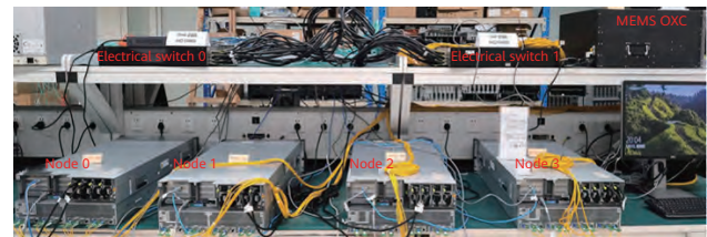
Figure 23 Prototype of an 8-server 64-NPU AI optical interconnection cluster
