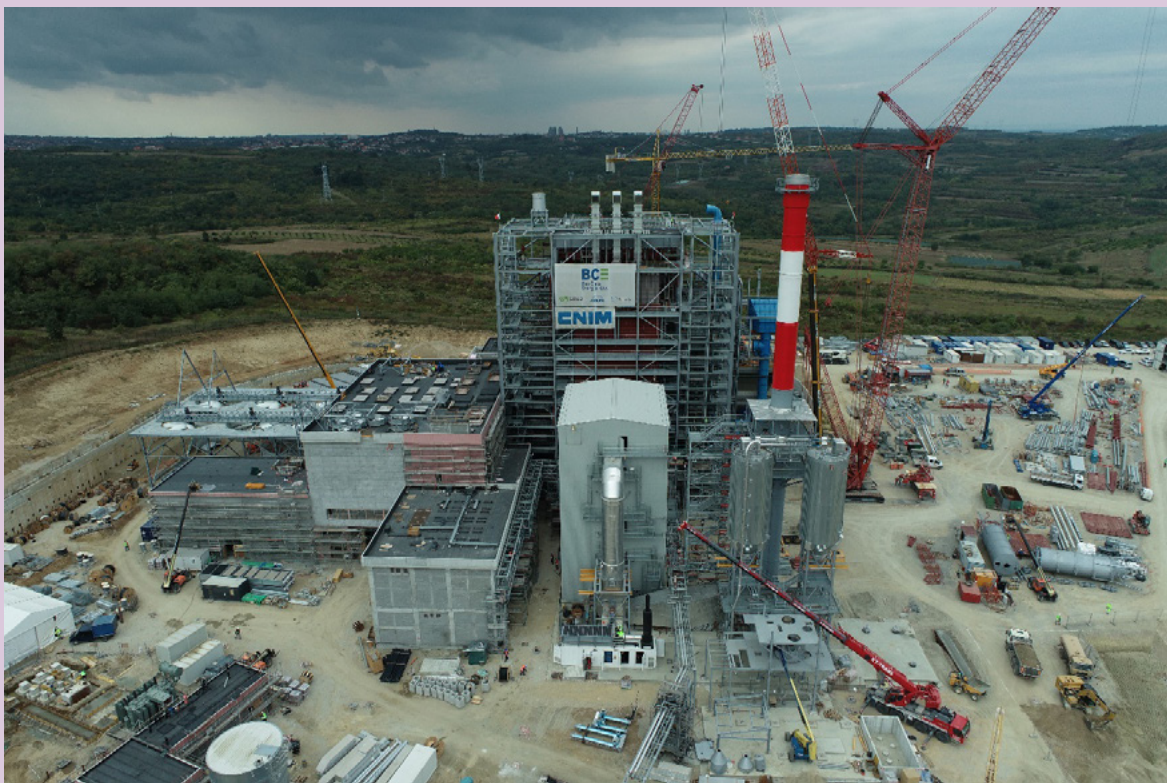
Work in progress on the Vinča landfill, June 2021. Photo credit: Beo Čista Energija
