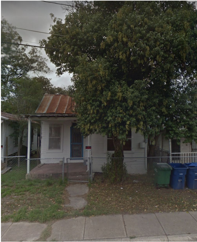
Potential Blight #3: Home in need of maintenance on S Smith St.
