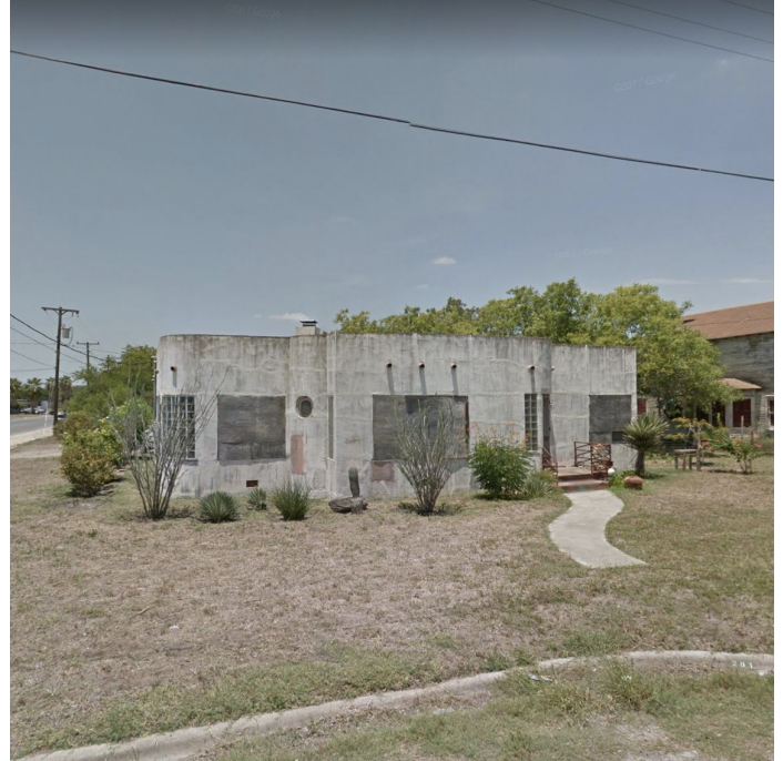
Potential Blight #2: Vacant Home on N King St.
