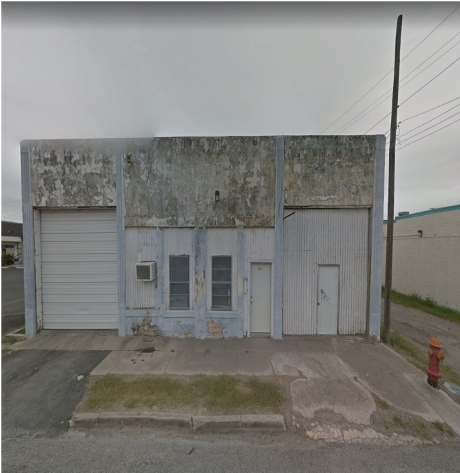
Potential Blight #1: Vacant Building on E 1st St.
