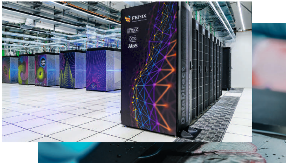
The TGCC computing centre of the French Alternative Energies and Atomic Energy Commission (CEA) is part of the Fenix infrastructure.
