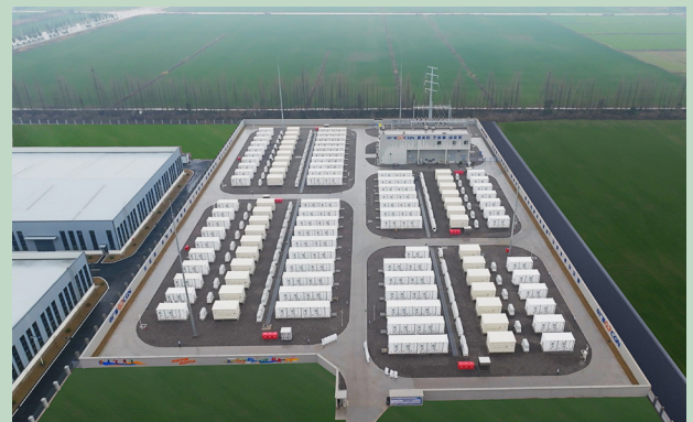
A 100MW BESS in China's Hubei project used Huawei's battery risk warning function
