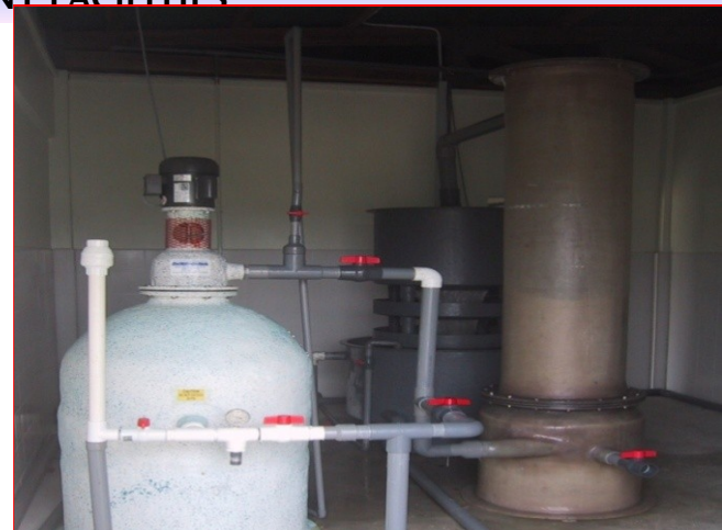
Sand Filter & Foam Fractionator
