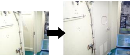
Development of Women’s Quarters (Installation of corridor doors in front of shower rooms on naval vessels)
