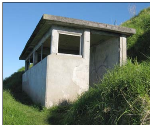
Figure C-6. 25: Extant example of the same type of BOP encountered at Crows Nest Fort. Located at North Head Battery, Auckland, New Zealand.
