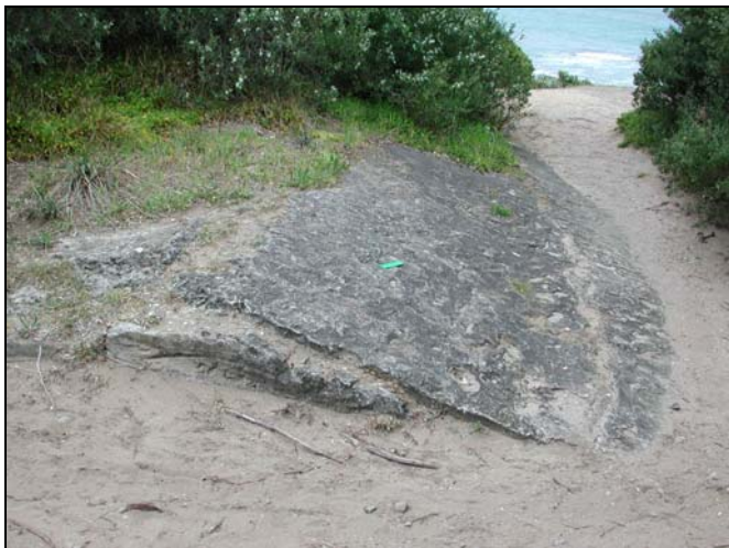
Figure C-6. 9: Exterior (formerly buried) apron of the 8" HP gun casemate, Crows Nest Fort (1886).
