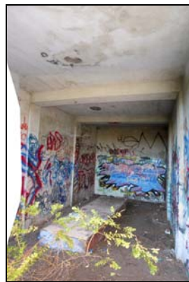
Figure C-6. 36: Pt Lonsdale generator bunker interior.
