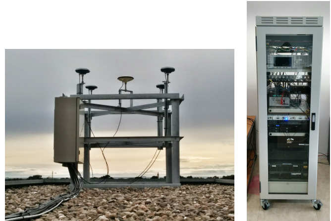
(a) Antenna platform.
