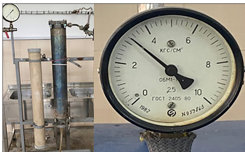
Figure 3. Column for cleaning sawdust with steam, T = 140\text{--}160\text{ }^{\circ}\text{C} , P = 2.5\text{--}3.2\text{ atm}
