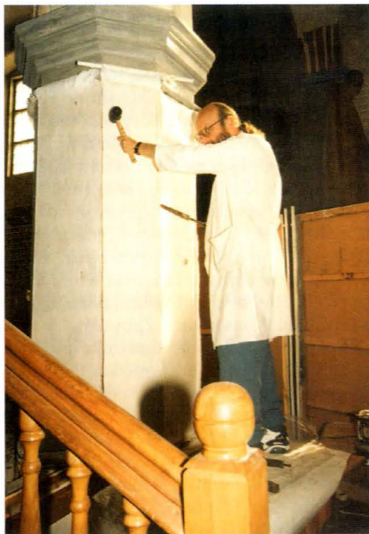
4. Filar pld.-wsch. w trakcie odcinania tynku od muru na pld.-zach. ścianie. Stan podczas konserwacji. South-eastern pillar during the removal of plaster from the south-west wall. State during conservation.
