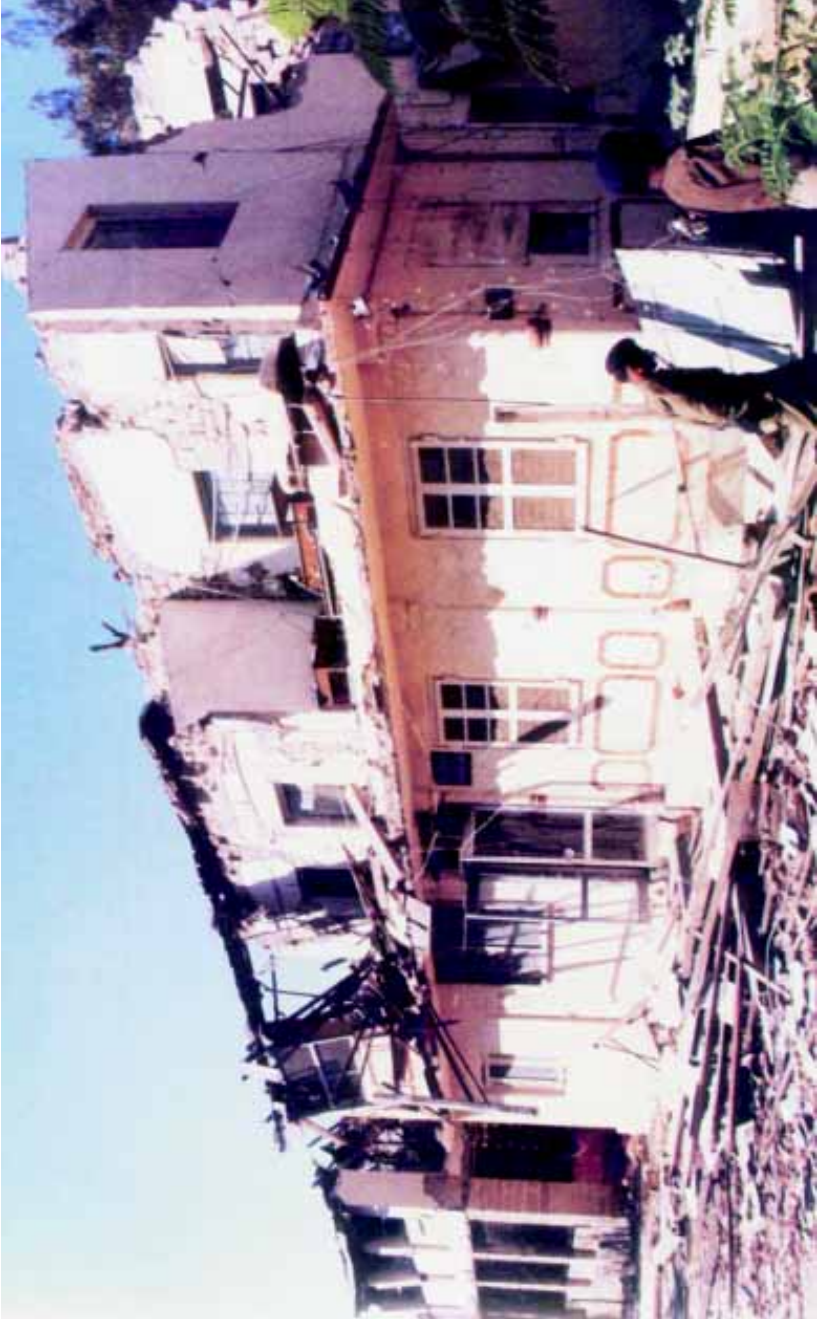
Damaged office of the Collector and District Magistrate at Bhuj
