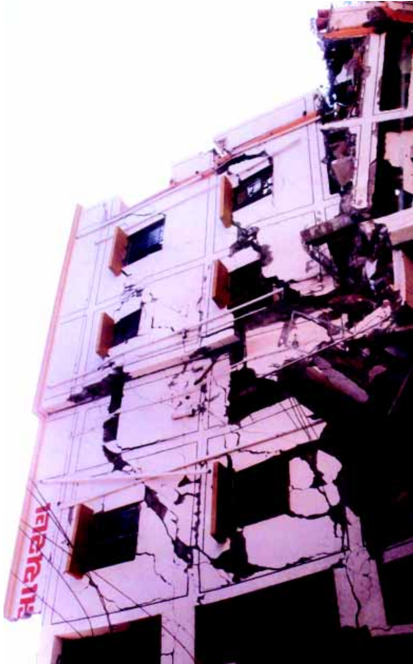
A collapsed building at Bhuj
