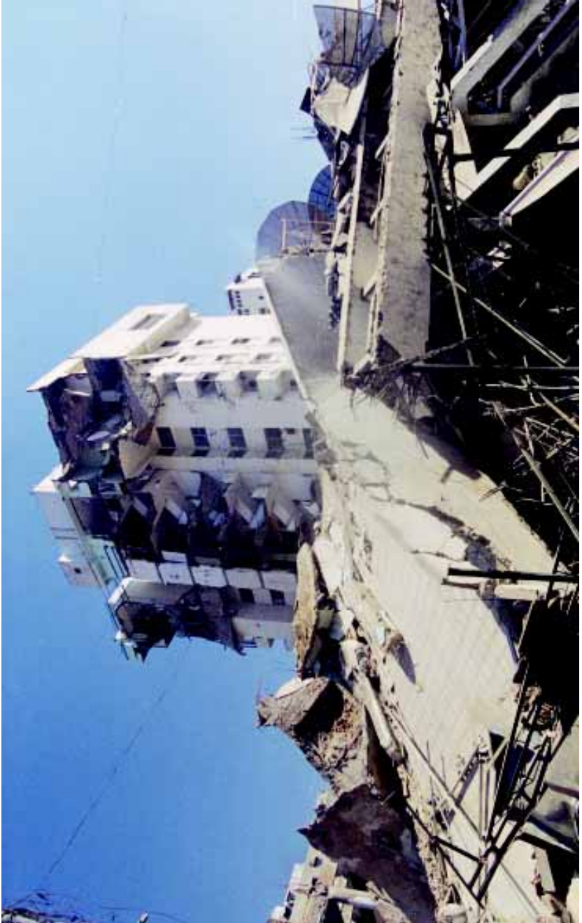
Damaged and collapsed apartments of Mansi Towers, Ahmedabad
