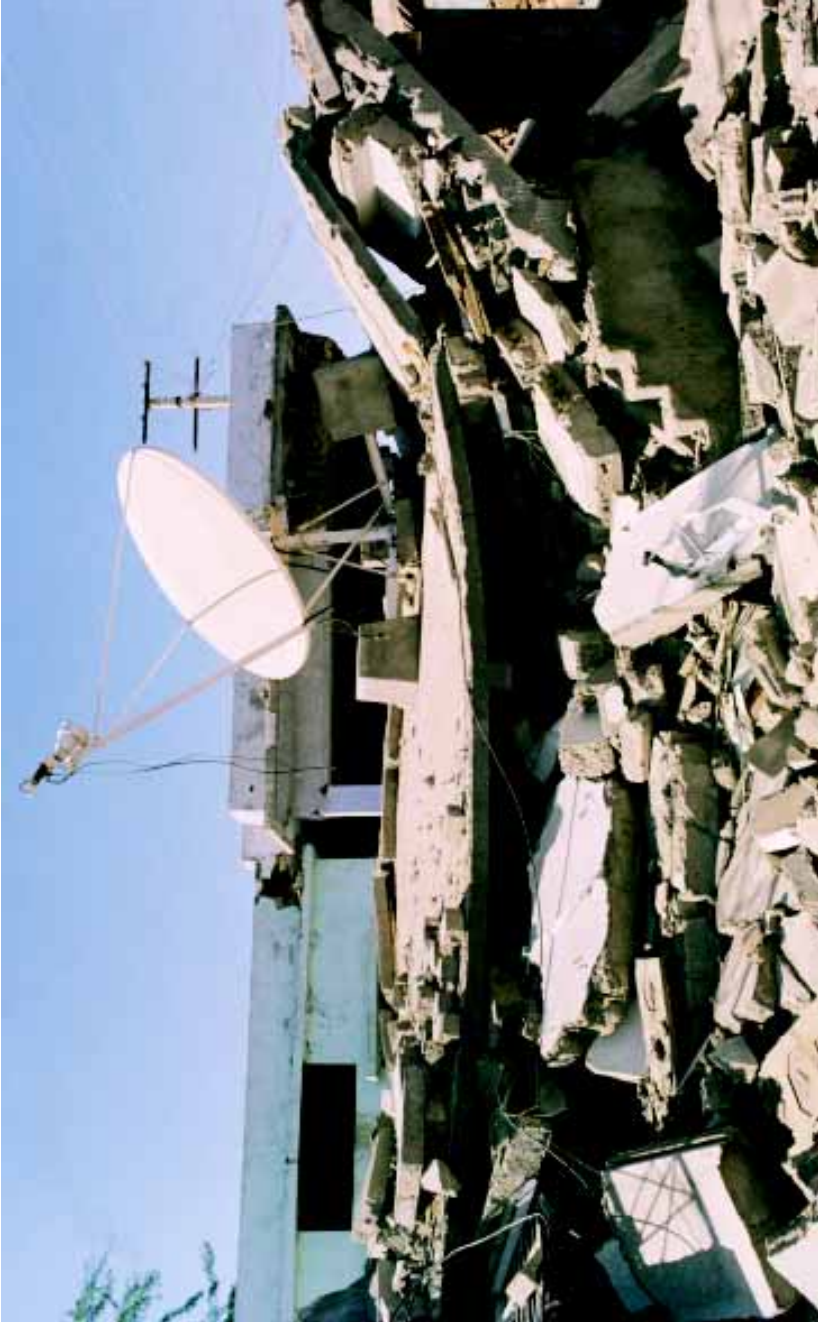
Damage to the telephone exchange in Khayda village
