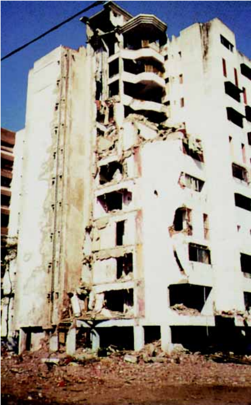
Damage to multi-storey Hare Krishna Apartments in Surat
