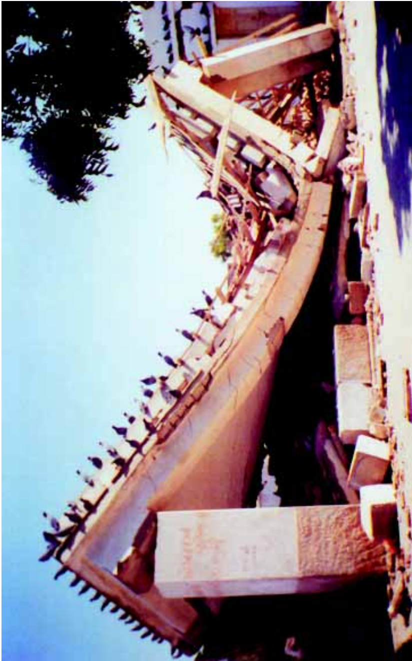
Collapsed newly constructed bus stand at Vondh village close to the epicentre of the earthquake
