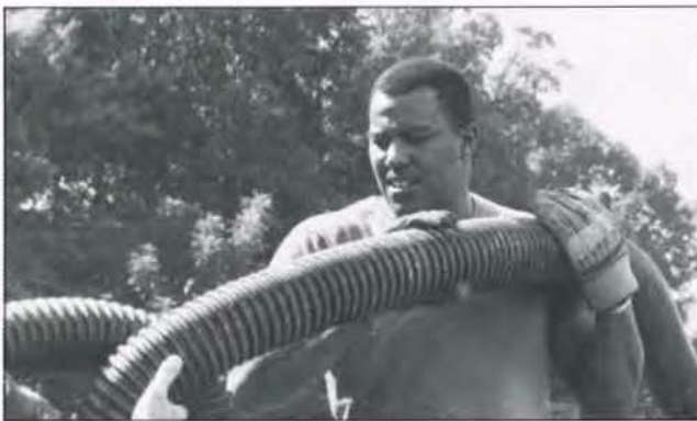
TWISTIN': Staff Sgt. Michael Lee Myers, 175th Civil Engineering Squadron, Maryland Air National Guard, wrestles with a snake-like length of flexible drain hose as a PRIME BEEF civil engineer unit installs a septic system at Montrose. (Photo by Capt. Mike Milord)
