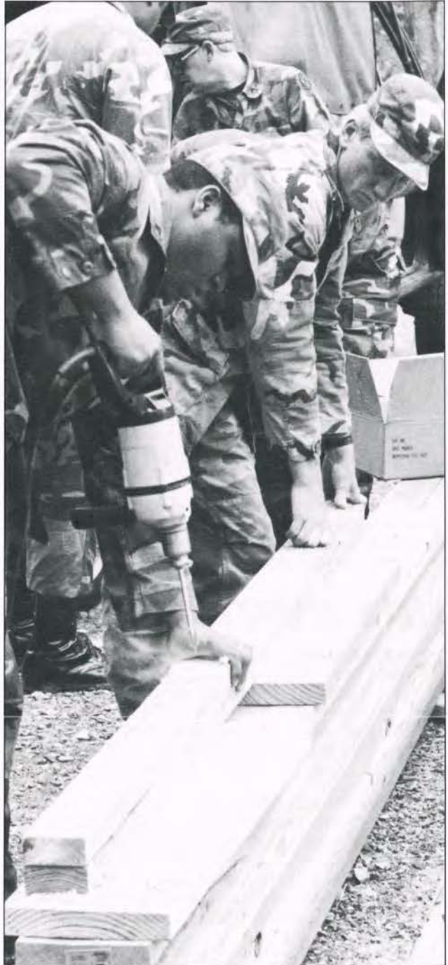
"BORE-ING": Sgt. Stanley Queen, Company A, 121st Engineer Battalion, Maryland Army National Guard, prepares framing by drilling holes in a 2"x4" as Sgt. Mark Merson, also of Company A, keeps it steady at the Savage River site of the 1989 Whitewater Canoe/Kayak Championships (Photo by Tom Darden, Governor's Press Office)
