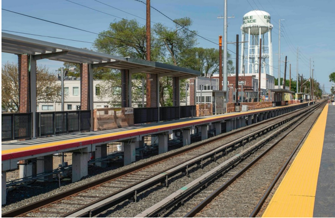
View east of the westbound Carle Place platform. Brickwork is being added to the canopy supports and permanent railings are being installed, May 17, 2020.
