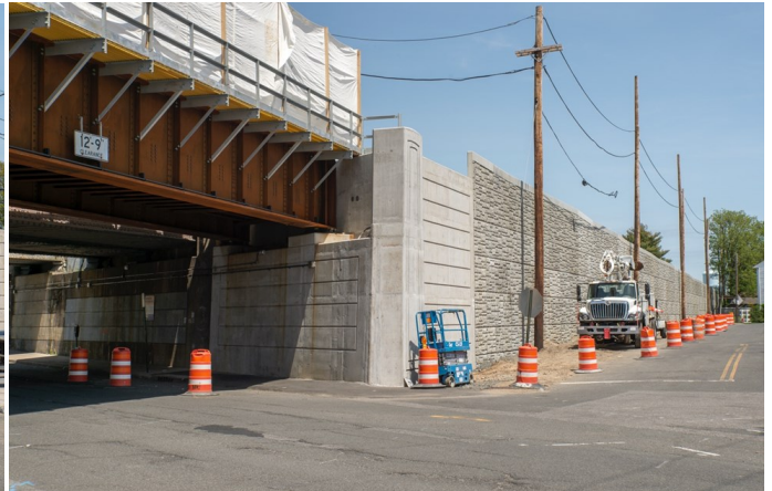
The architectural finishes of the new bridge abutments match as closely as possible those of the original bridge abutments from the 1962 grade crossing elimination project. The combination retaining wall and sound barrier extending to the right are also newly constructed.
