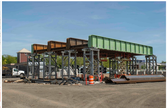
The new three-track bridge has already been built and is awaiting installation, scheduled for the weekend of June 6-7.
