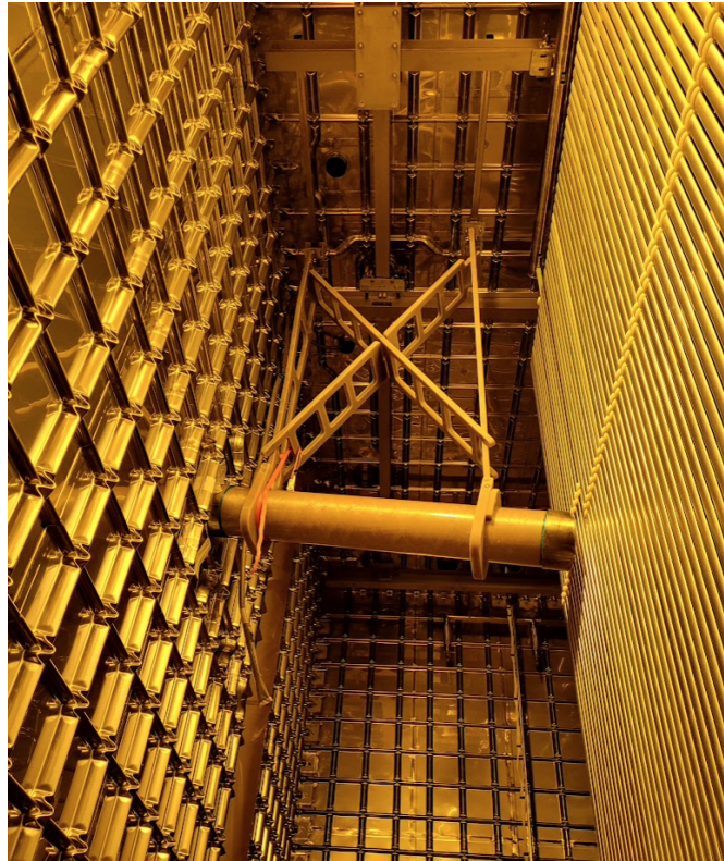
Figure 8.14: Photo of the beam plug realized and installed in the FD1-HD Module 0
