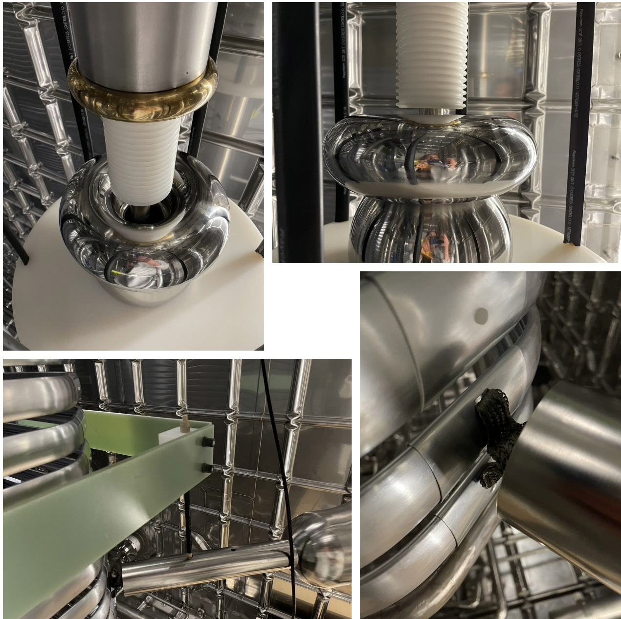
Figure 5.4: Components of the full scale HV long-term stability test in the NP02 cryostat. Top: two views of the doughnut and the sphere of the extender head with the HVFT tip connected. The gold colored ring in the top left photo is the sleeve to confine the gas bubbles produced by the heat input from the HVFT and evacuate them to the gas phase close to the HVFT ground skin. Bottom left: the tip of the extender in front of the field cage. Bottom right: Detail of the extender connection to the field cage.
