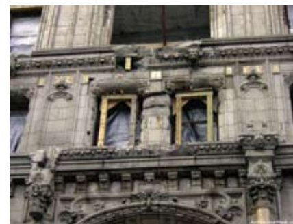
Grand prize for his year's Prism Stone in Architecture Awards went to the restoration of the 90 West Street Building, New York, designed by Cass Gilbert.
