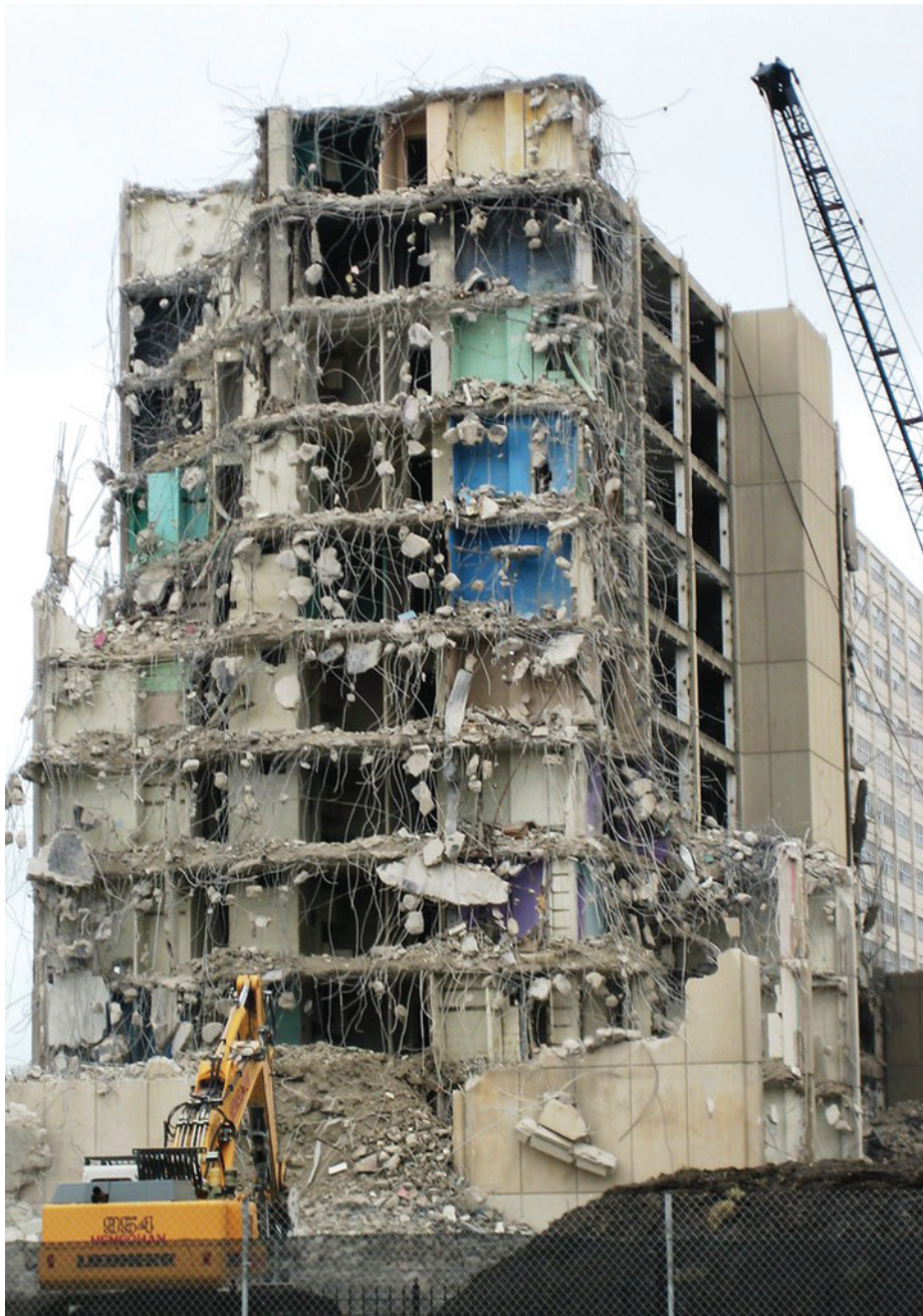
Demolition of the Cabrini-Green high-rises took years, and the final building came down in late March 2011. APARTMENT THERAPY / FLICKR
