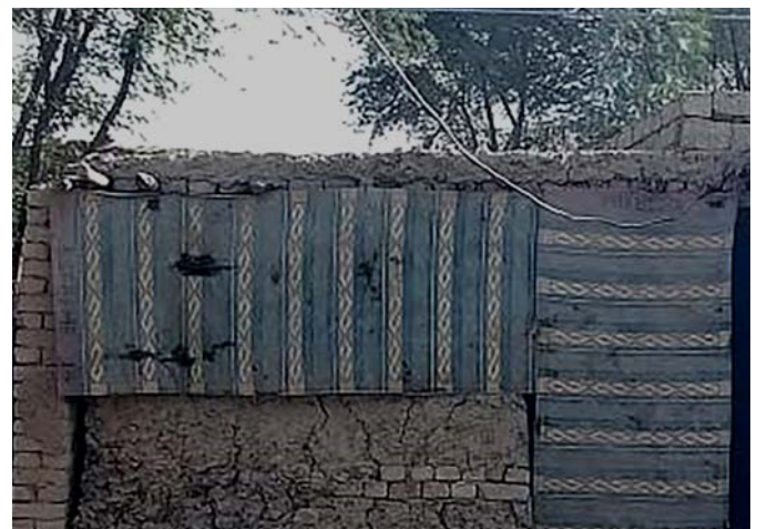
Figure 3. The condition of the housing of family 2. Picture A Overall housing condition. Picture B rooms damaged during the flood.
