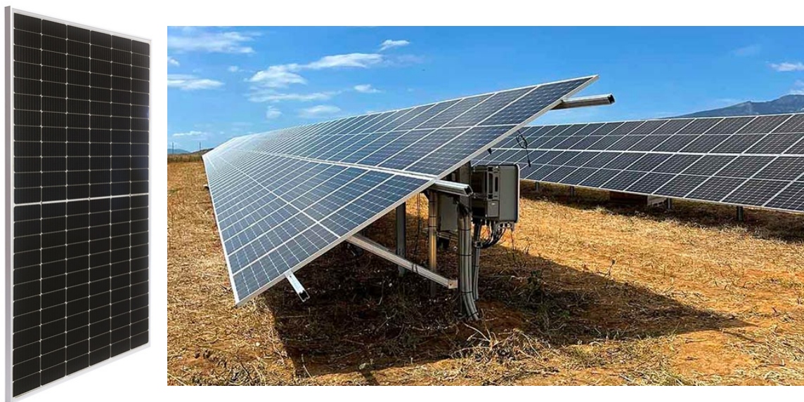
Figure 6: Picture of FU 460 M Silk Pro module and its use in a utility scale pant (courtesy of Futurasun).
