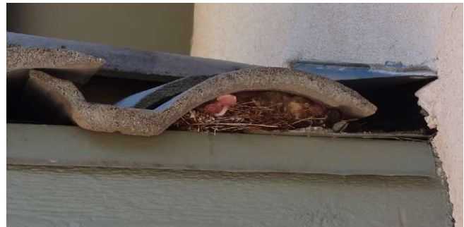
Figure D17: The ends of the barrel-tile roof covering on this home were not “bird-stopped.” Note the debris in the under-roof area at the end of the roof (lower photograph). Source: IBHS.
