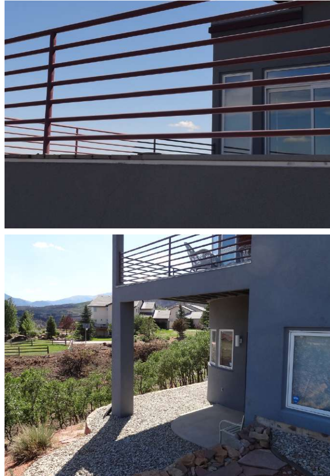
Figure D23: The decks at this home used wood for the structural support system and a combustible wood-plastic composite decking (walking surface) product. Source: IBHS.
