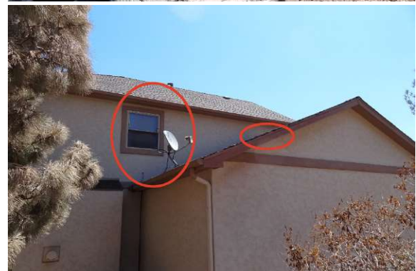
Figure 18: A composite figure of two damaged homes on the west side of Courtney Dr. The up-slope home is above and the down-slope home is below. The charred combustible siding in the up-slope home is not visible in this figure. The damaged components in the down-slope home are circled. Source: IBHS.
