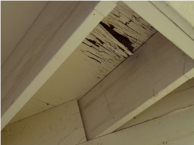
Figure D19: The flagstone covering on this solid surface (noncombustible) deck had failed (upper) allowing water to get below the covering, eventually resulting in fungal decay in the horizontal wood-based sheathing (lower). Source: IBHS.
