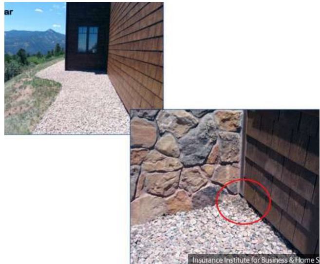
Figure D5: The upper left photograph depicts the vegetation management (defensible space) at the rear of the house. The lower right photograph shows an accumulation of dried vegetative debris in the corner, on top of the rock mulch. Source: IBHS.
