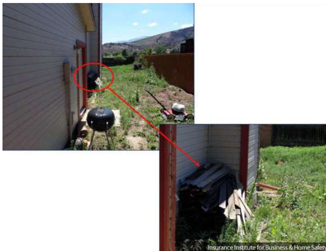
Figure 27: Combustible materials were present in the near-home zone of the Champagne Drive home. Source: IBHS.
