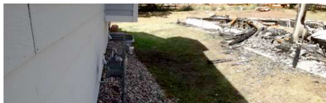
Figure 11: The distance between the destroyed home on the left and the damaged home on the right was approximately 16 feet. Source: IBHS.
