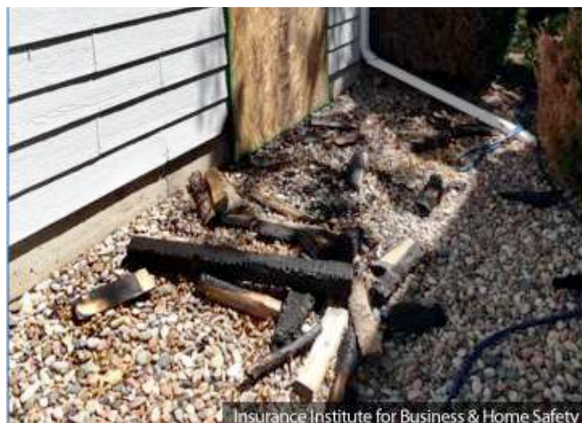
Figure 12: Embers ignited a firewood pile located next to the garage of this home. The direct flame contact exposure from the burning firewood ignited the composite wood (hardboard) siding product. Source: IBHS.
