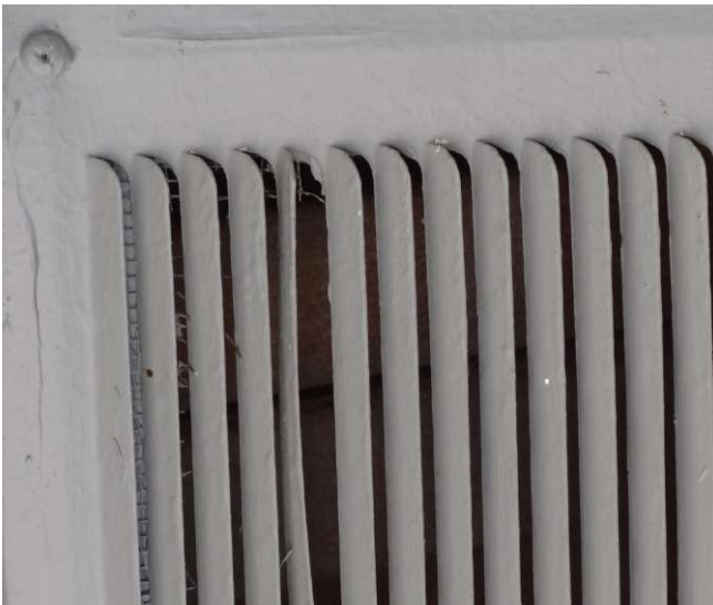
Figure D16: A soffited eave was used on this home. Some of the under-eave vents did not have mesh screening. Source: IBHS.
