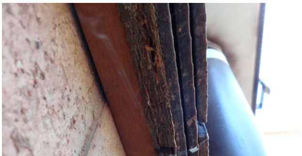
Figure 21: The siding on this home was a noncombustible fiber-cement shingle product (upper photo). The assembly at the base of the wall, showing combustible wood-based sheathing, is shown in the lower photo. Source: IBHS.
