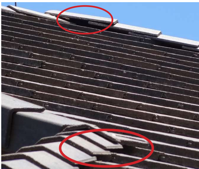
Figure D8: Un-stopped/unblocked openings at the hips of the flat-tile roof. Source: IBHS.
