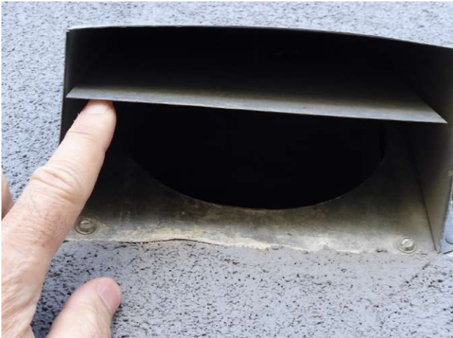
Figure D24: Dryer and other exhaust vents used vents coverings that were normally closed (upper left); when operating positive pressure in the duct would force open the closure flame to at the outlet. Source: IBHS.
