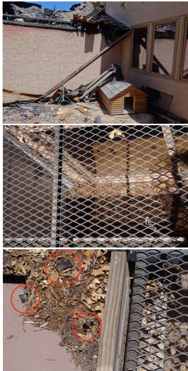
Figure 26: Combustible materials were present in the near-home zone of the Rossmere Street home. Embers are evident in the right-hand middle photo (embers circled in red). Source: IBHS.
