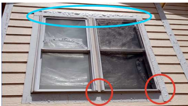
Figure 13: Radiant heat from the burning home, which was destroyed and was located 20 feet from this damaged home, was sufficient to cause paint on the wood trim to bubble (circled blue) and thinner components on the vinyl window frame to deform (circled red). Source: IBHS.
