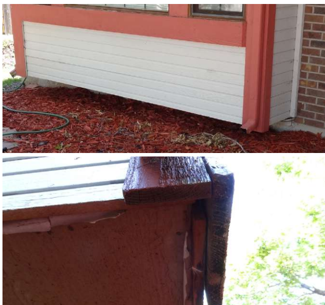
Figure 28: The "bump out" design feature at the front of the Rossmere Street home would be been vulnerable, if the wood mulch had been ignited by the observed ember exposure. Given the low earth-to-wood clearance, flame spread to the bump out would have provided a flame contact exposure to the combustible underside feature. Source: IBHS.
