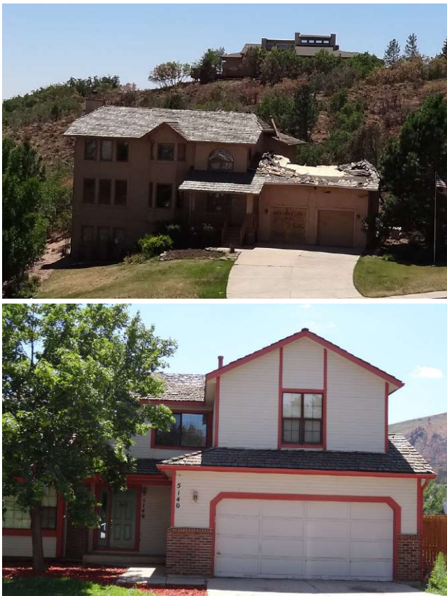
Figure 25: Homes on Rossmere Street (upper) and Champagne Drive (lower), each had wood shake roof coverings that were ignited by wind-blown embers. Source: IBHS.
