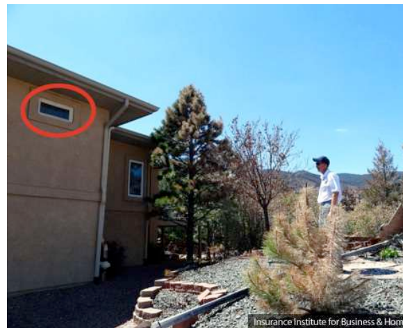
Figure 7: This damaged Talleson Court home was approximately 30 feet from a destroyed home. Two windows were damaged (one is circled in red; another window of the same size is located to the left of the one shown). The tall pine tree had lower branches removed and noncombustible gravel was used within approximately 10 feet from the house. Note the scorch on the destroyed home side of the pine tree and small tree in the foreground. Source: IBHS.
