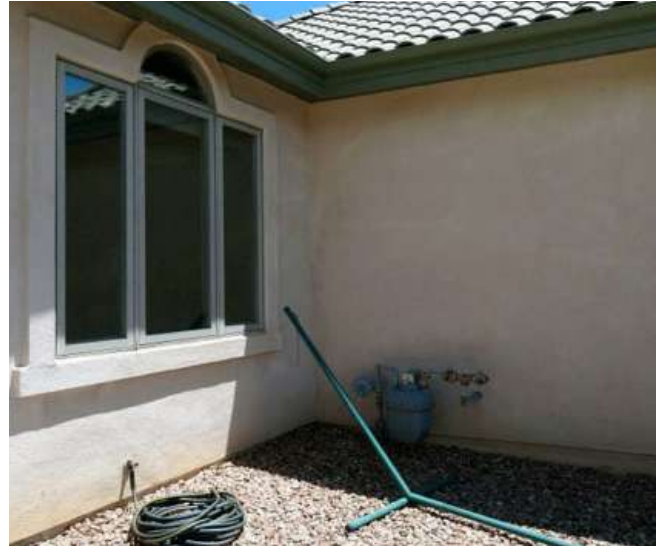
Figure D15: The defensible space in the near-home zone on the right side of the home was good. Source: IBHS.
