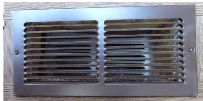
Figure D7: These photographs show venting for the make-up air to a room containing gas appliances. Metal screening was missing from these vents, as seen in the lower photograph. Source: IBHS.
