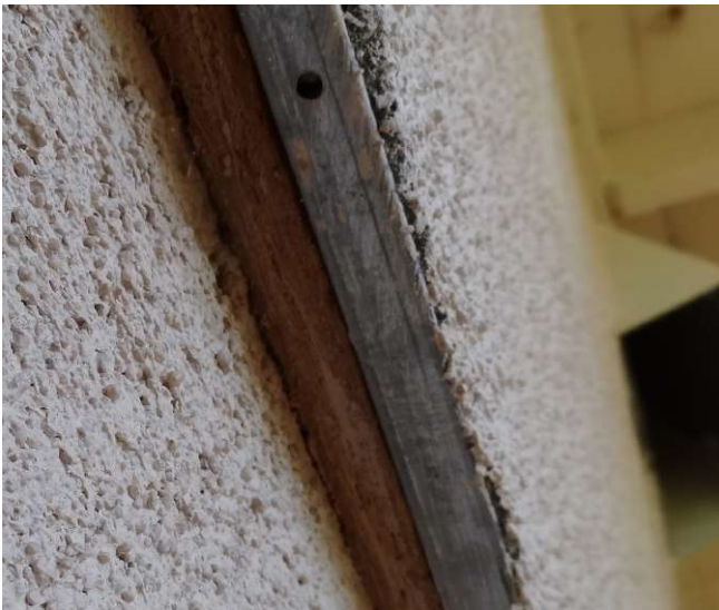
Figure D14: Bark mulch was used in areas at the rear of the home, under one of the decks. Note that the wood-based sheathing product is exposed (lower photograph). Source: IBHS
