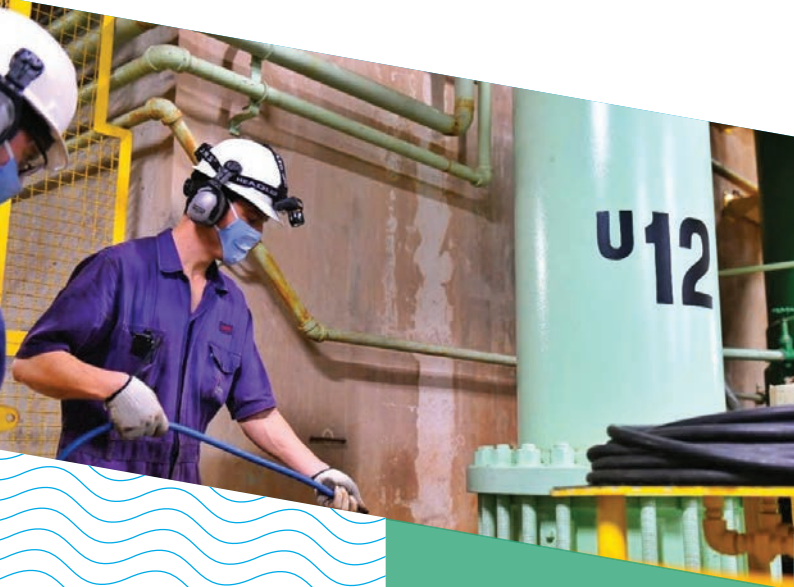
Photo: Engineers at the Itaipu hydropower plant, between Brazil and Paraguay, continue maintenance operations while applying strict new Covid-19 health and safety guidelines. Credit: Itaipu Binacional
