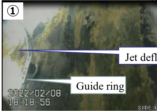
Installed at 6:18 PM on Feb. 8
