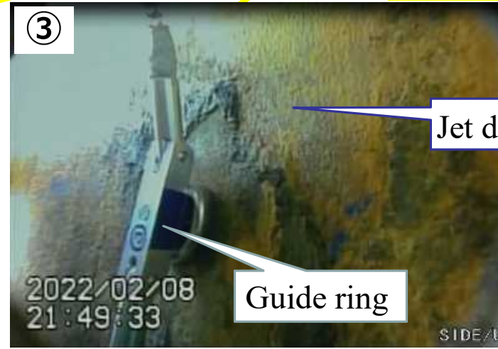
Installed at 9:49 PM on Feb. 8
