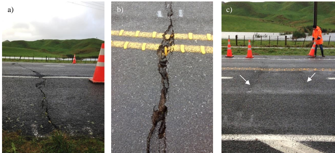
Figure 1: Observed damage to the road. a) North crack; b) Detail of the north crack; c) South cracks, as indicated by the arrows.
