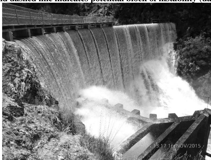
Figure 4b: Present day overtopping event at No.2 Dam (taken from downstream of right abutment, November 2015).
