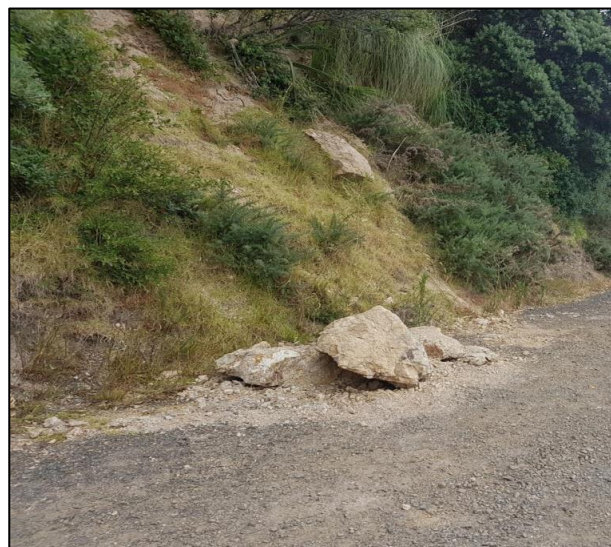
Figure 8: Fallen blocks on footpath
