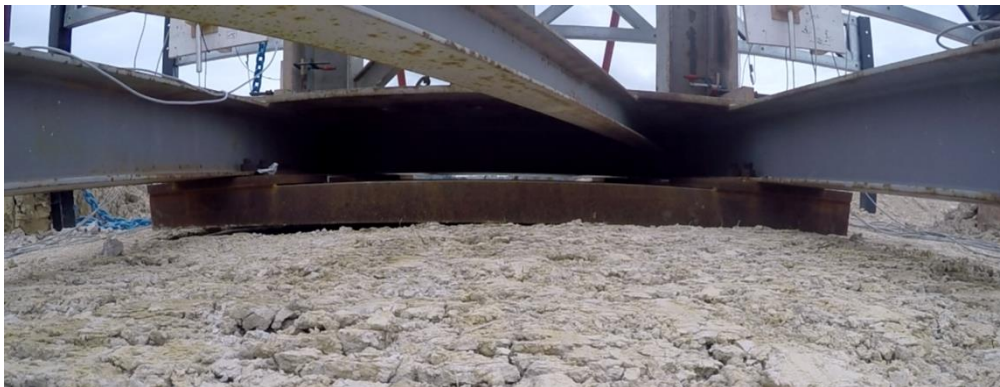
Figure 5: Partial detachment of the footing with the underlying soil
