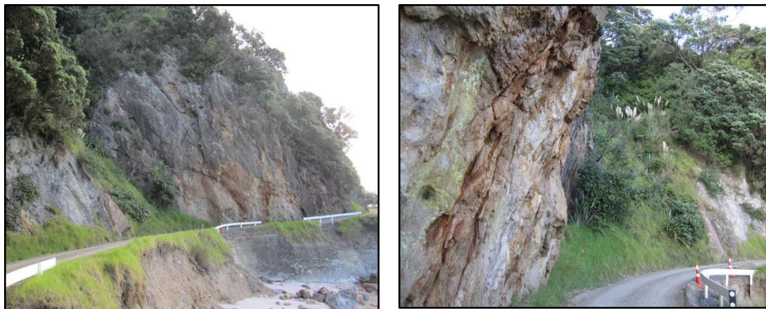
Figure 2: Views of Bluff Road section of concern showing overhang, fracturing and weathering/alteration
