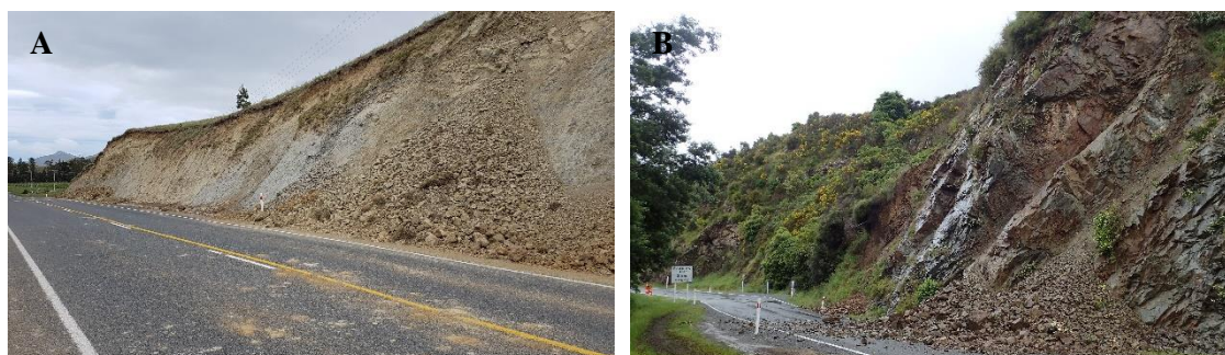
Figure 4. Examples of cut slope failures along SH1. (A) Failure of low height cutting in weak Tertiary siltstone, with accumulation of debris over the lower part of the slope. (B) Failure of cutting in indurated greywacke bedrock with encroachment of debris onto the road.
