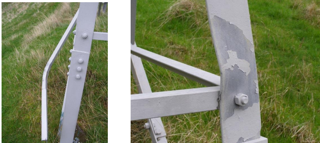
Figure 2: Examples of rock damage to pylon
