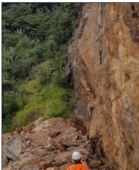
Figure 7: Open fractures above path
