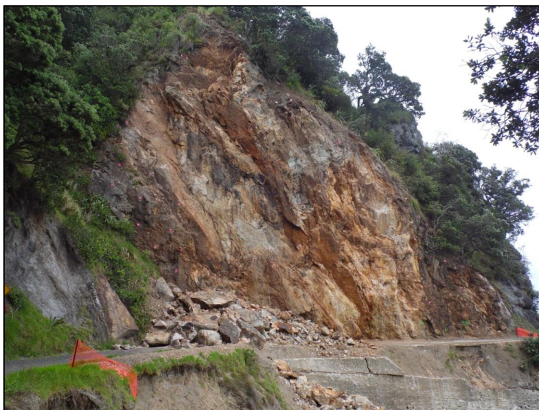
Figure 4: Rockfall of 25 December 2015.
