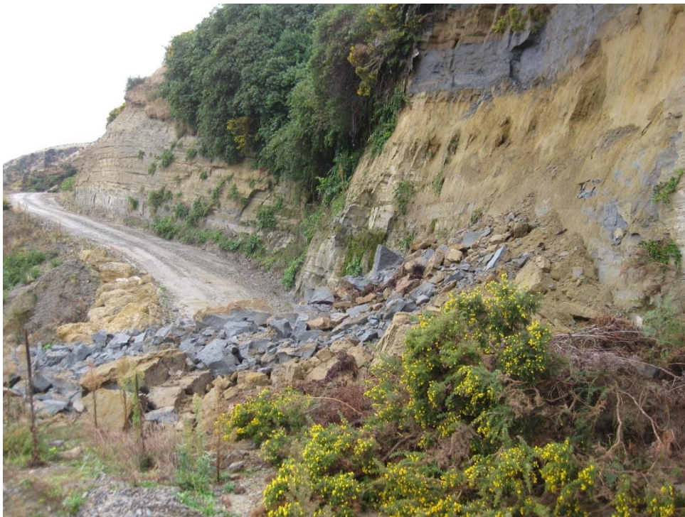
Figure 3: Slip in 2010, debris extending over the access road
