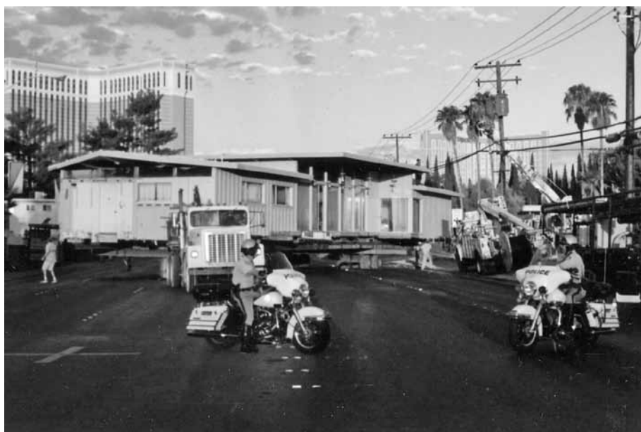
Morelli House being moved down Fremont Street, 2001. Photographer unknown. ( Special Collections Department, University of Nevada, Las Vegas )
