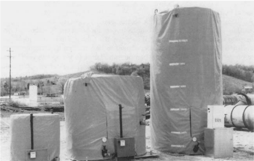
Figure 7 Insulated tanks for holding liquid fat at feeder lots. Note thermostatic controls for electrical heater (bottom center of each tank) and waterproof vinyl-coated covers. Courtesy of Griffin Industries, Cold Spring, Kentucky.
