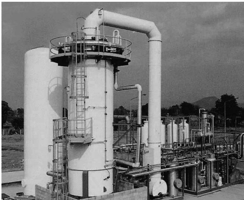
Figure 6. Steam/Methane Reforming Plant HYDRO-CHEM Processing, Subsidiary of Linde AG. (This figure is available in full color at http://www.mrw.interscience.wiley.com/biofp .)
