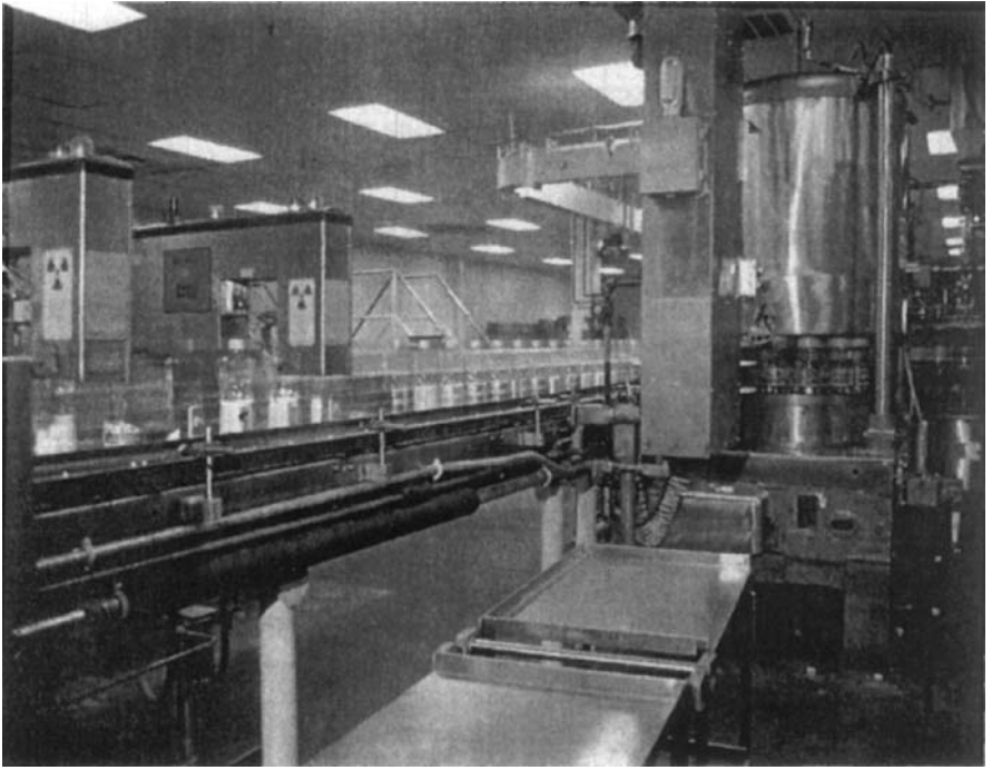
Figure 4. Liquid oil filling line.
