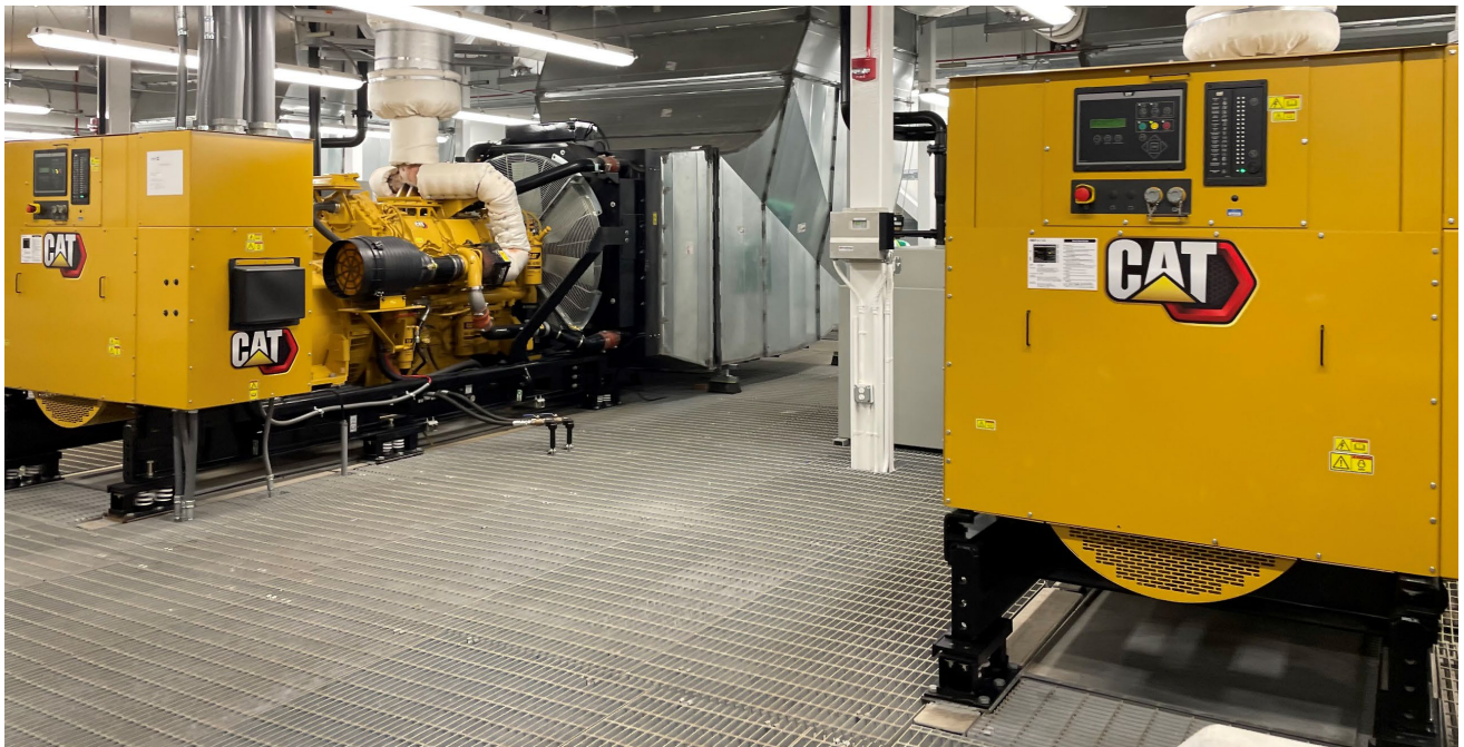
New generators at the Wilcox Medical Center on Kaua'i add redundant capability in case of power outages, Jan. 25, 2022
