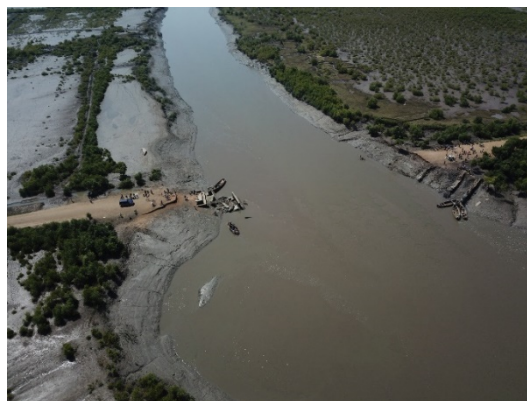
Watercourse erosion leading to collapse of bridge
