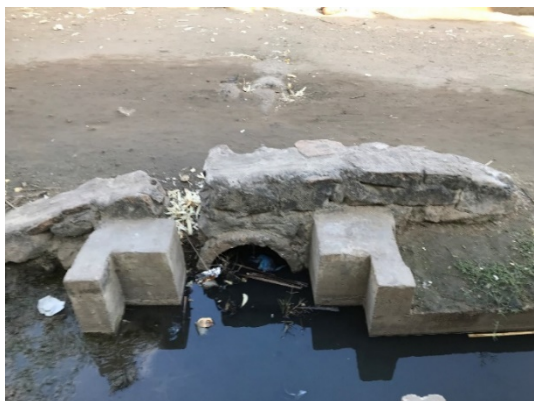
Insufficient drainage / waste management
