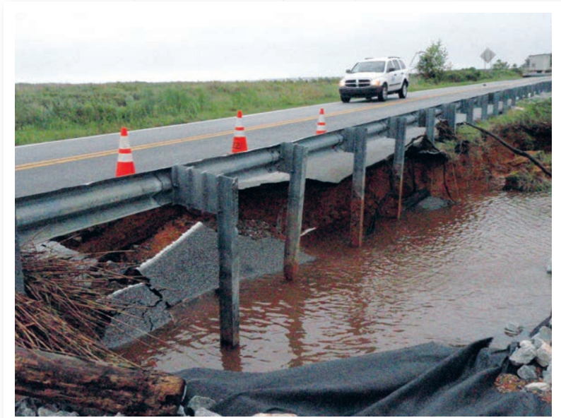
The impacts of storm surge from Hurricane Irene in August 2011 take a toll on State Highway Route 9 over Augustine Creek near Port Penn, Delaware.
