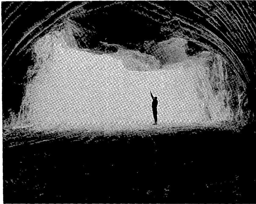
Fig. 3. Tunnel deformation of surface-ramp entrance.
