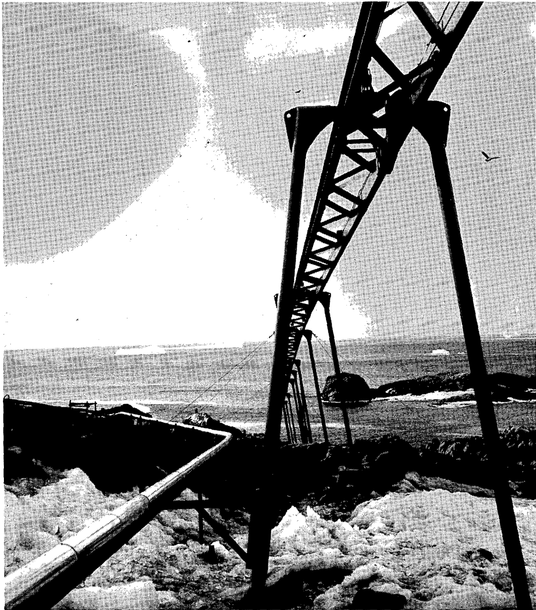
Discharge pipework for waste water and hot brine outlet following the course of the refuse monorail.
