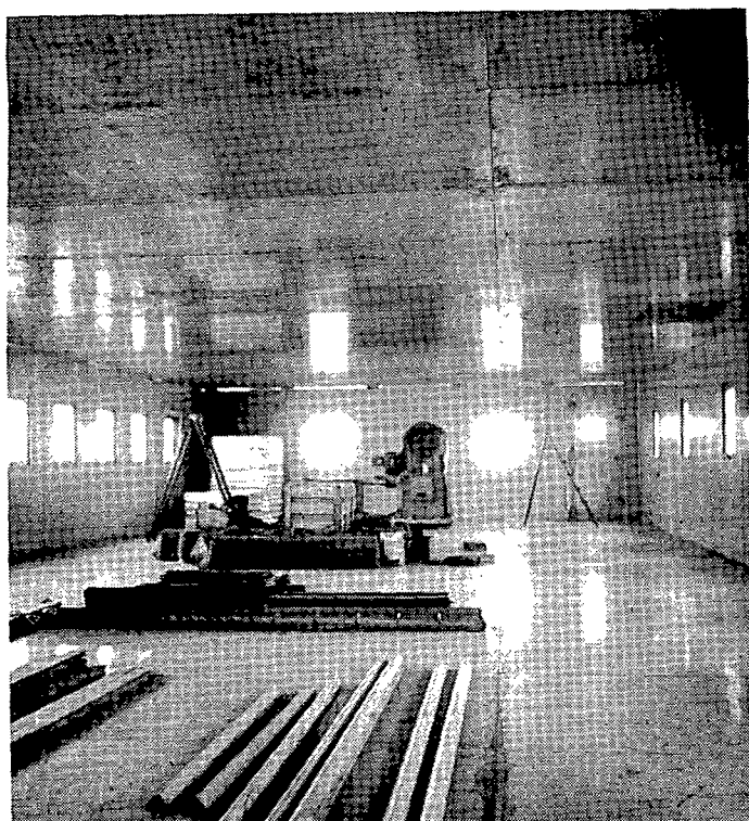
Photo 5. Inside view of a laboratory building after laying of panels and before assembly of the prefabricated metal partitions. Neither beam nor post; surface and volume are free for all installations. Weather proofing and joint covers are not yet laid. In the background; hot-air generator.
