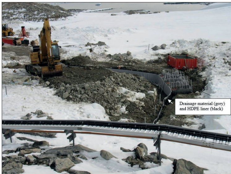
Photo 2: Installing wings and gate. Note: gate is heavily instrumented for research purposes.
