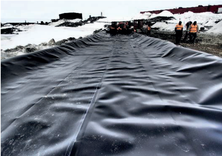
Photo 3: Geomembrane (black) installed over GCL and berms. Note the heat welded seam running through the centre of the geomembrane showing two panels joined together.
