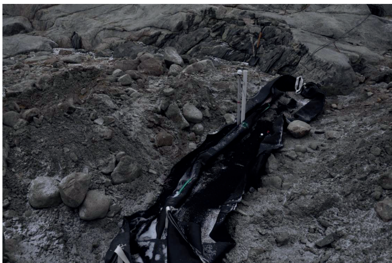
Photo 6: PRB gate installed using geotube (black fabric). Note: once operational the top covers are closed to prevent granular media dispersing into the environment.
