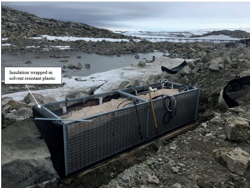
Photo 4: PRB gate being constructed using “cage pallet” showing piezometers (white tubes) for water monitoring and sequenced granular reactive media. Black wire is heat trace to be connected.
