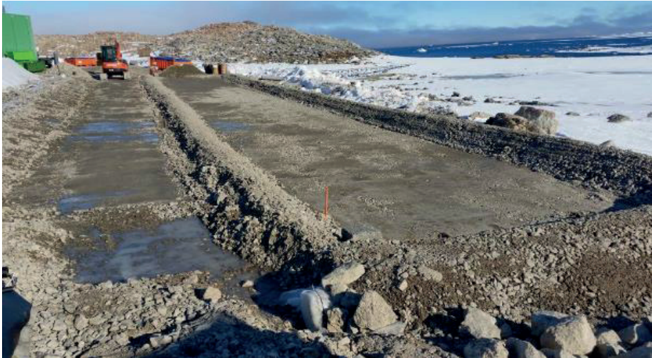
Photo 1: Compacted biopile subgrade with earthen berms prior to installing the other components of the composite liner system (geosynthetic clay liner, geomembrane and geotextiles).
