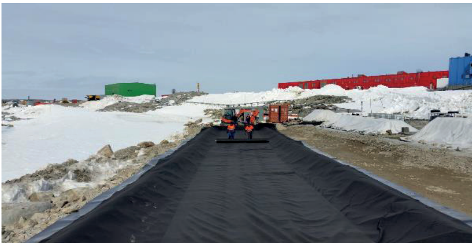
Photo 4: Completed construction of the composite liner system showing geotextile (black) overlaying geomembrane (black/grey) and GCL below.
